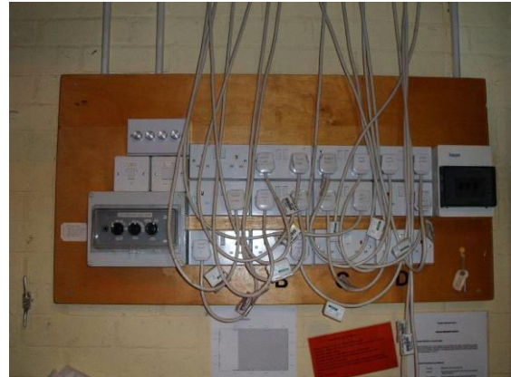
Figure D.3 Remote controlled distribution panel
