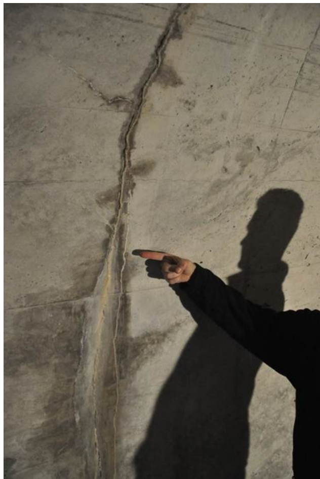
Fig. 2.3: Example of seepages inside the tunnels.
