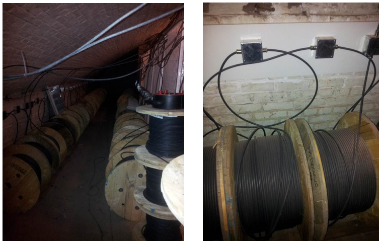
Figure 6.26: Nexans cable on their drums
