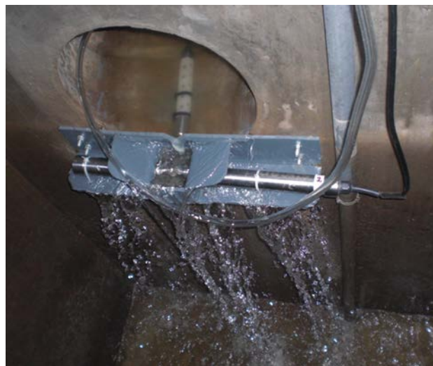
Figure 49: s::can probe at the inlet of second batch feeding system
