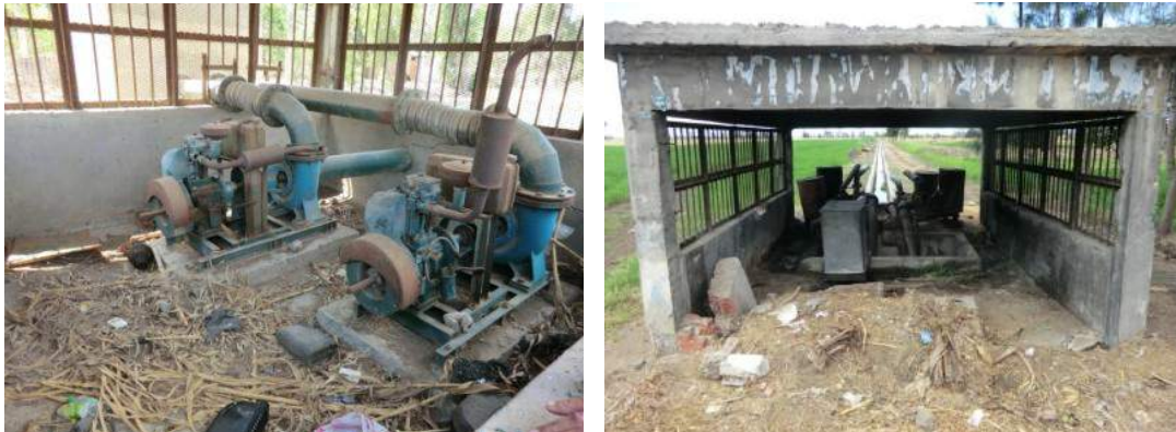
Figure 11. Unused pumps (left), individual pumps using the pit (right) (Ariamon)
