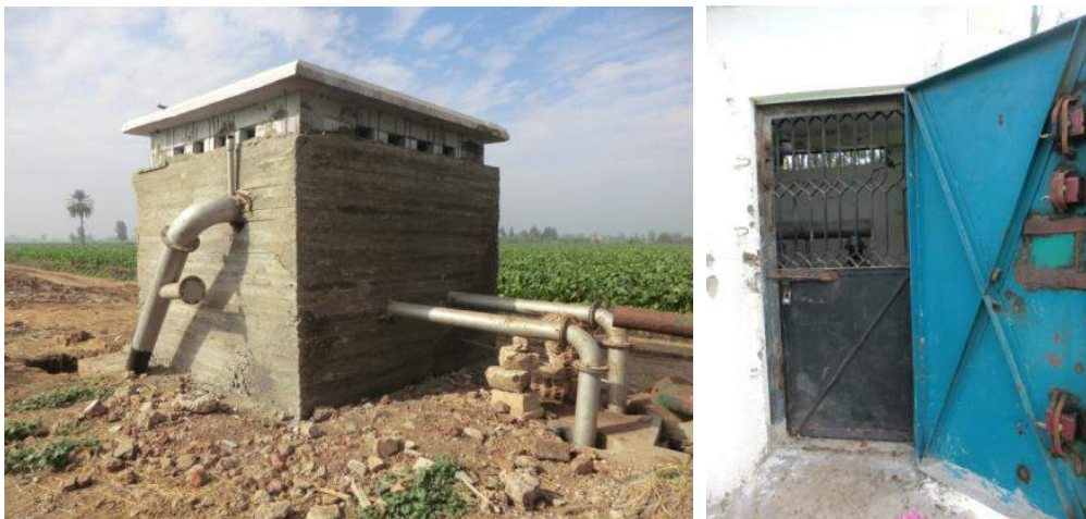
Figure 9. Pump station with a reinforced concrete protection
