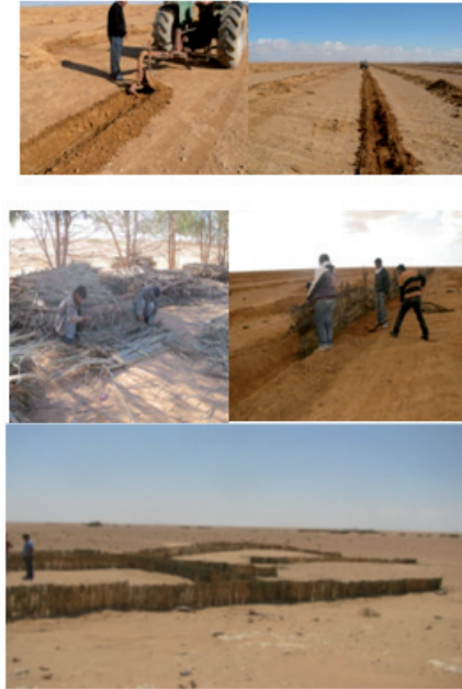
Figure 8. Site preparation for the project area and implementations of sand dunes fixation by
