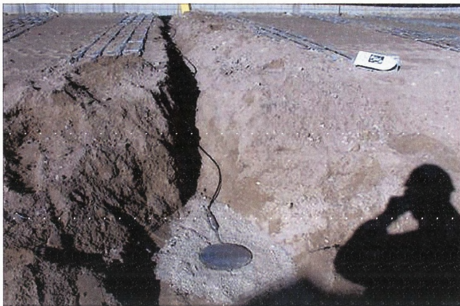
Fig. 3.7 Photograph showing an installed total pressure cell before burial
