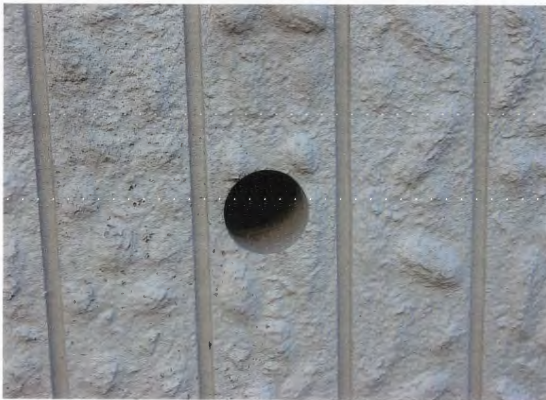
Fig. 3.17 Hole cored in secondary stage concrete fascia panel to allow access (Inclinometer H2)
