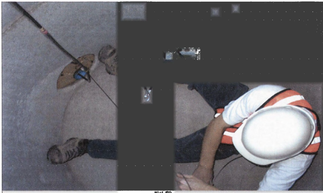
Fig. 3.9 Photograph showing the inside of the manhole where horizontal inclinometer No.1 (H1) is located
