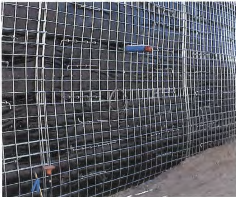
Fig. 3.10 Photograph of horizontal inclinometer No. 2 (H2)
