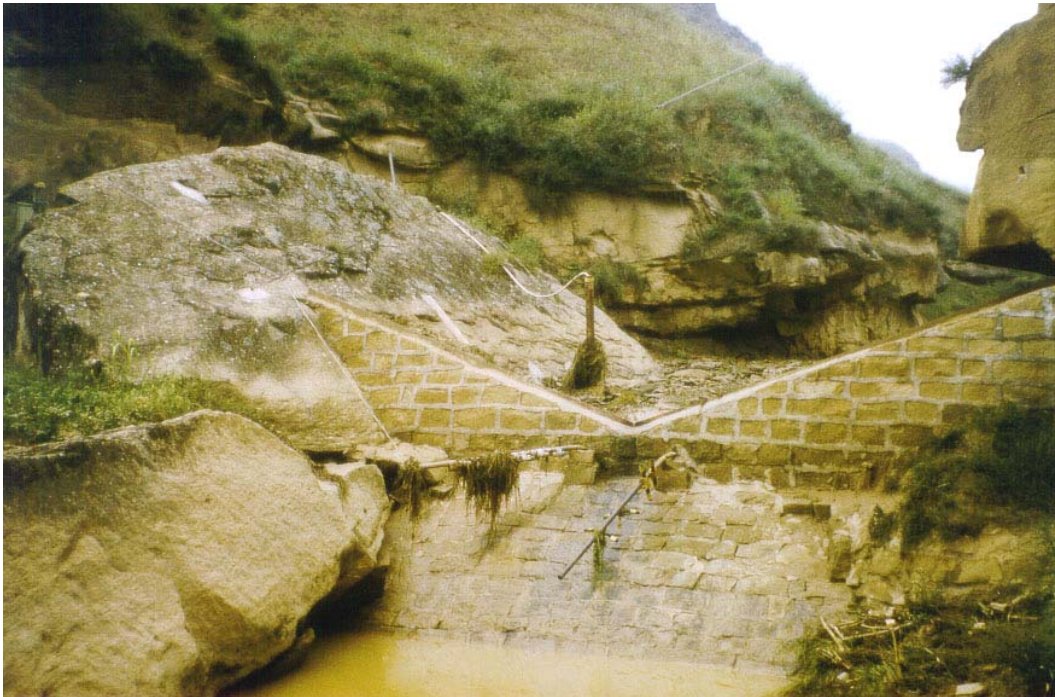
Figure 4.8 The weir on August 30 th , 2000. The supporting construction of the ultrasonic water level sensor as well as the sensor itself were destroyed by the event of 000829. Note the large amount of plant material around the pipes and around the pipe of the pressure transducer (background). Water level during the event was close to the top of the V-shaped weir.
