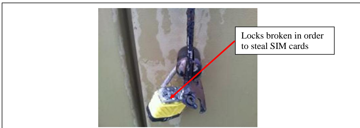
Figure 11: Vandalism of locks at mini substations in Sandton
