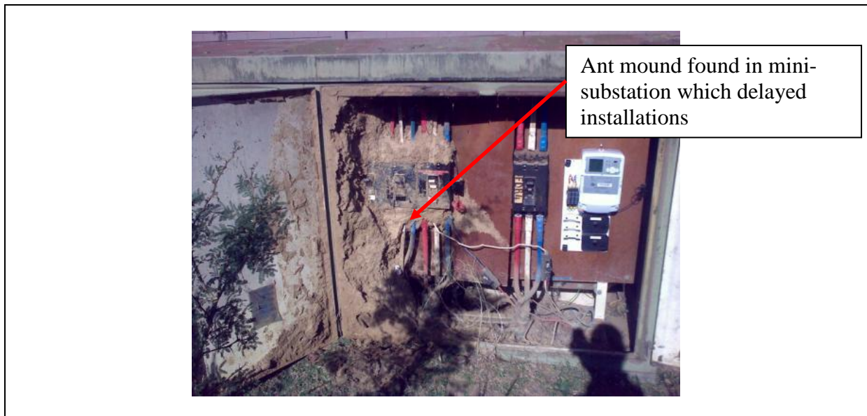
Figure 9: Ant mound in transformer mini substation in Sunninghill
