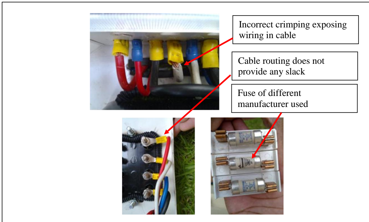
Figure 7: Poor quality field installations experienced in Sunninghill
