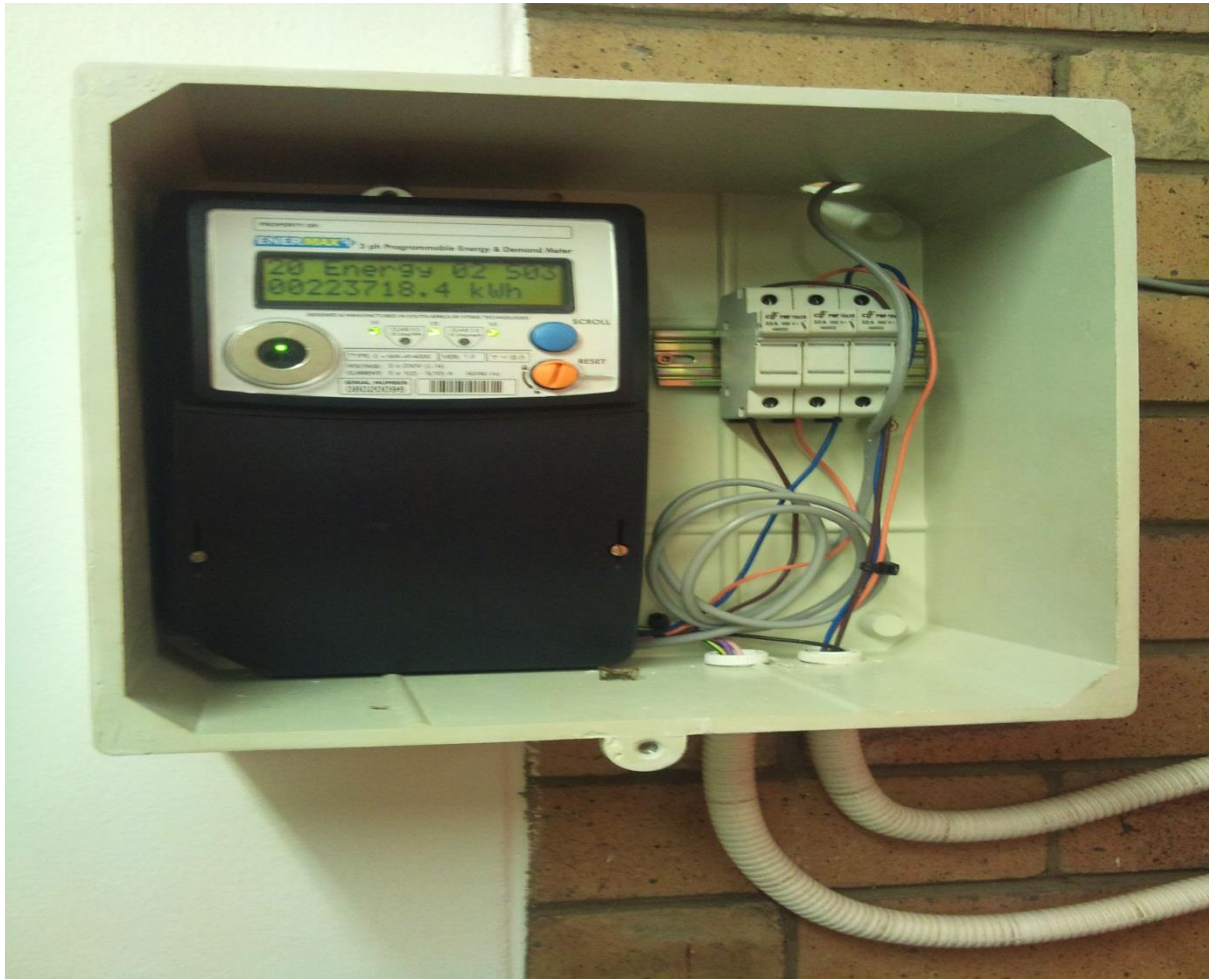
Figure 6: Digital Meter Reading (D J du Plessis Building Wits University)
