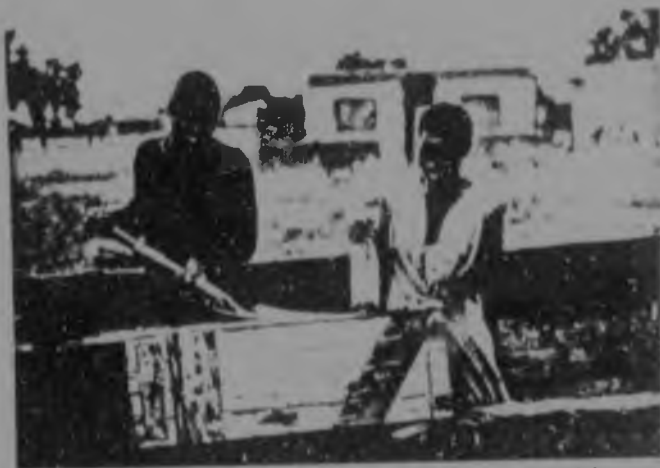
6a. Winterveldt: Member of the household assisting a contractor with building a rammed-earth wall.
