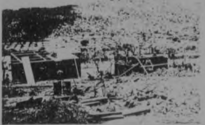
51h. While a brick-laying team completes its work on one house, a roofing team works on the one next door.
