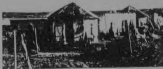
36a. A timber framework is built over a thatched roof prepared to be covered with sheet-metal.
