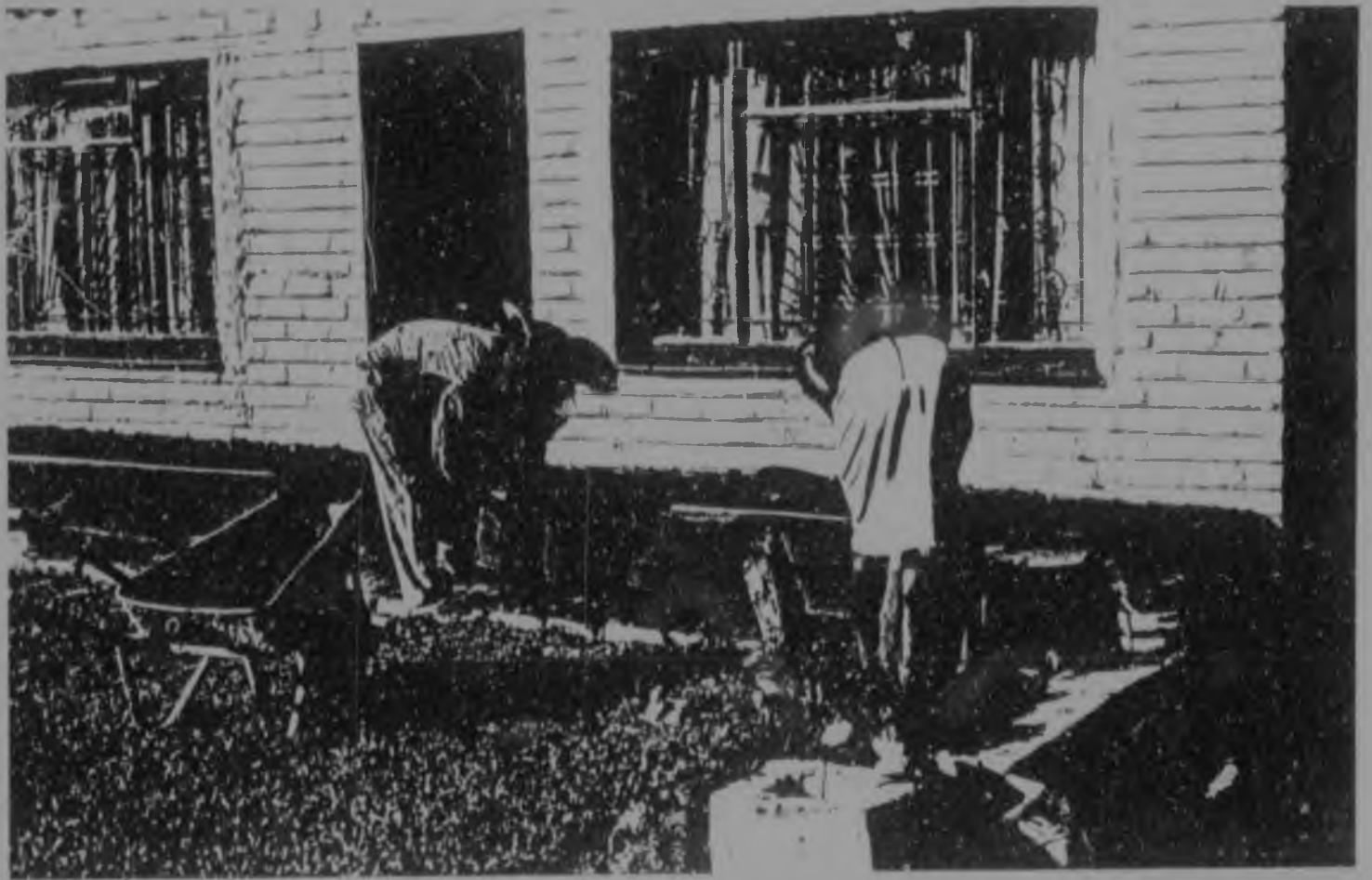
9c. kaNyamazane: A member of the household assists a contractor to build a bench against the front wall of a standard house-type. The windows were changed from those originally provided with the house.
