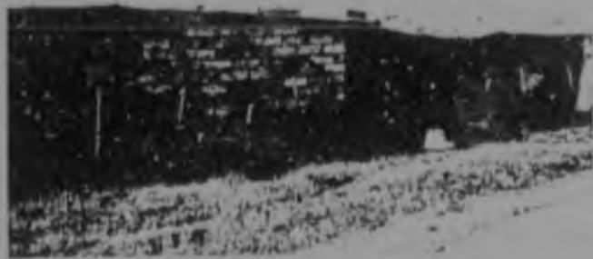
36e. Sand-cement blocks replace a piece of mud-wall that collapsed after heavy rains
