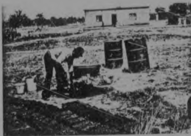
6d. Winterveldt: Contractor hired to make sand-cement bricks next to the building-site.
