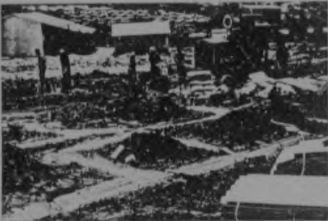
51e The Administration Board supplies concrete for foundations from a mobile concrete mixer.
