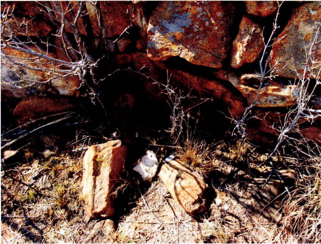
Figure 11: Large stone slabs were used to create a foundation to bear the load of higher walling.
