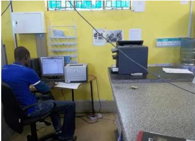
FIGURE 10: ONE OF THE FREQUENT USERS OF CONNECTIVITY AND THE POOR ELECTRICAL CABLING
