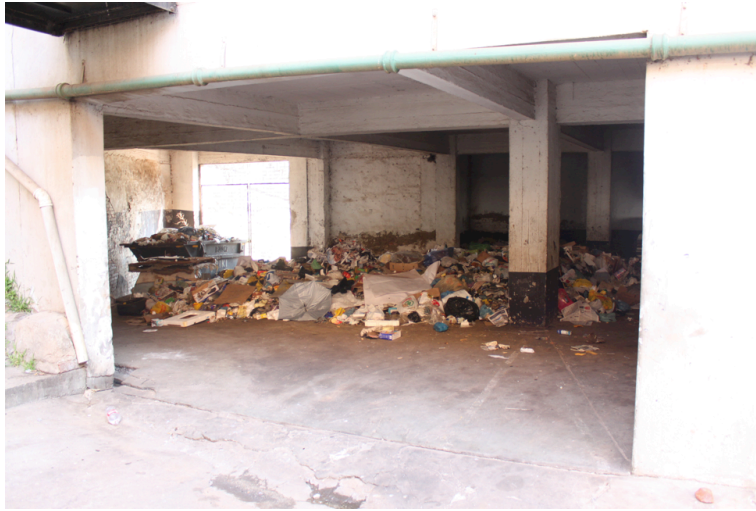
Figure A2.15: The ground floor parking garage where large amounts of rubbish began to be stored during a municipal rubbish collector's strike, and which seemed to grow due to there being too few bins for the building. The area was a haven for rats and children were told to avoid it. (Source: author's own photograph, June 2011).
