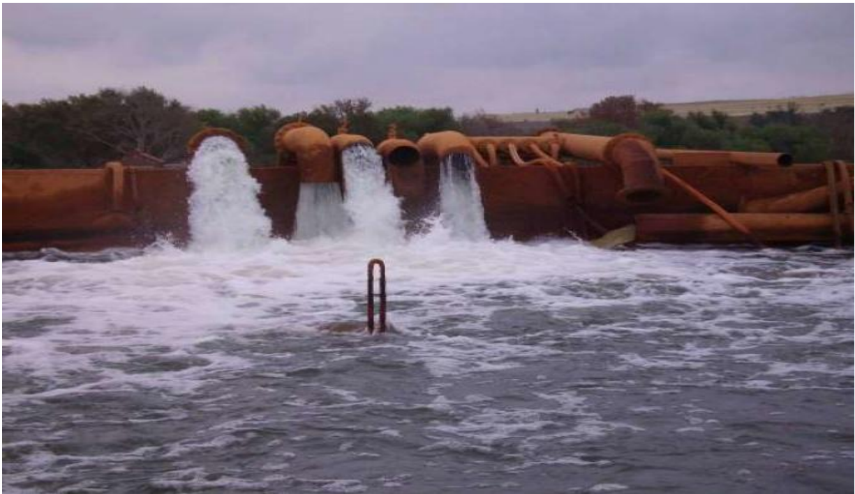
Figure 1.3: Water pumped from the Eastern Basin to the treatment plant at Grootvlei Min Source: Report to the inter-ministerial committee on AMD, 2010
