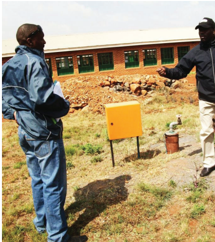
PHOTOGRAPH 16: Borehole which had been installed at a school yard vegetable growing project. This borehole and its pump have never worked.
