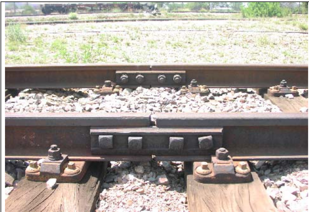
Figure 2.7: Nut and bolt jointed rail in South Africa
