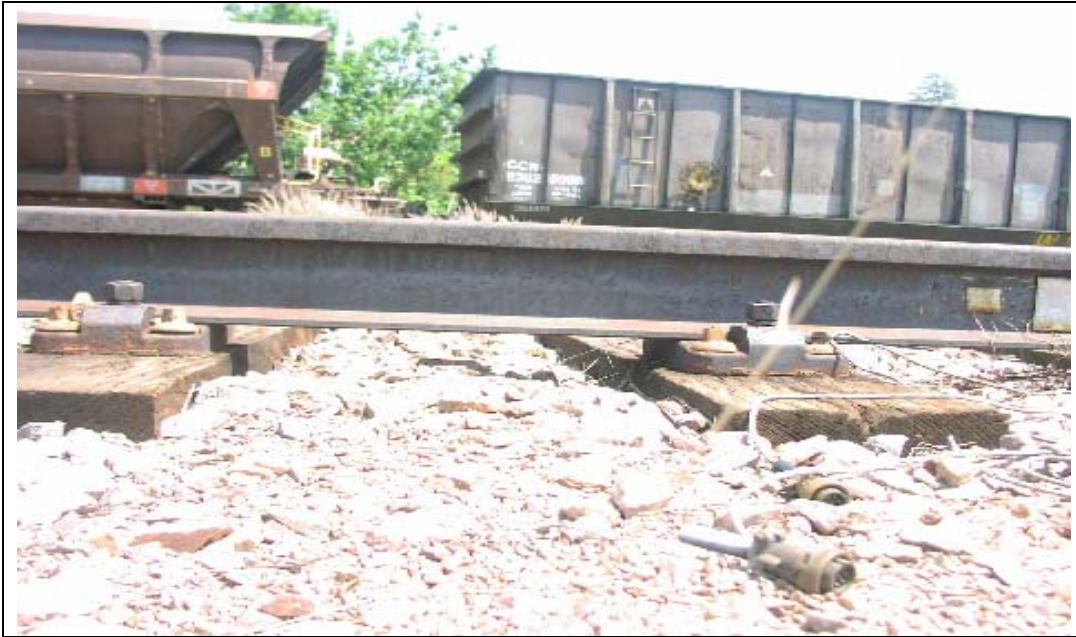
Figure 0.4M: Gap under straight and jointed rails.
