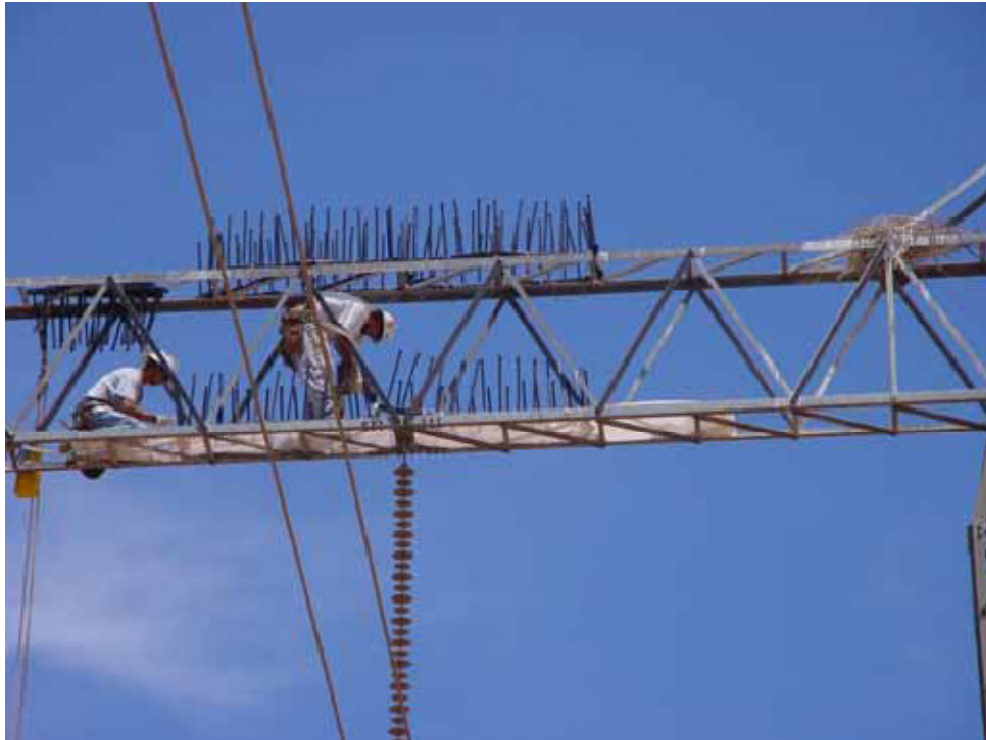
Figure 9 Installation of bird guards above phase conductor (Vosloo H. F., 2004)
