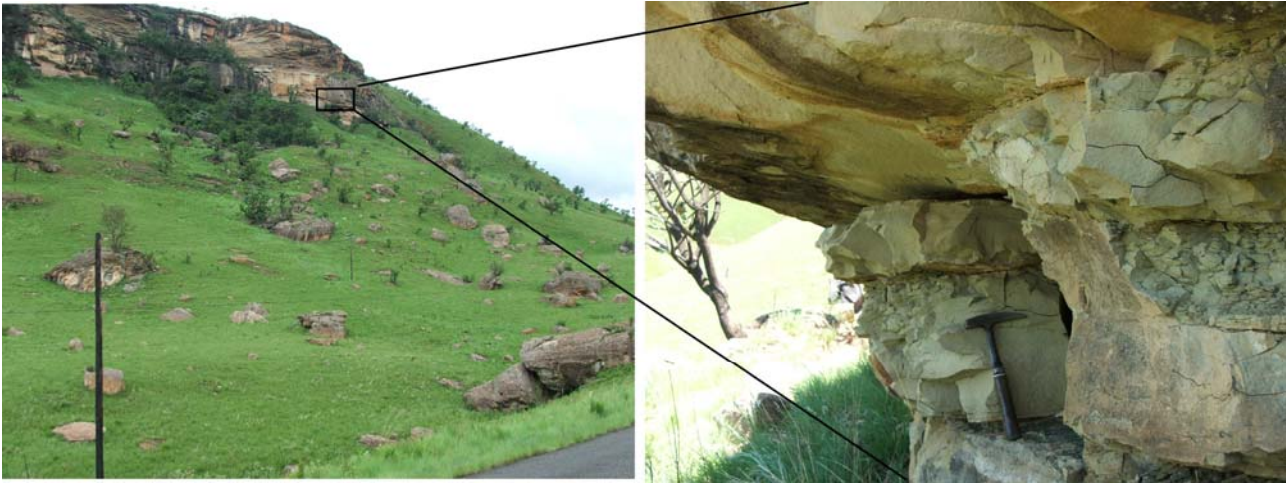
Figure 9. Rockfalls are a typical occurrence in the Drakensberg. Weathering of an argillaceous layer below a resistant sandstone bed or enhanced groundwater seepage results in formation of a hanging block of sandstone. Disengagement of these hanging blocks from the rock face is along fracture and joint planes
