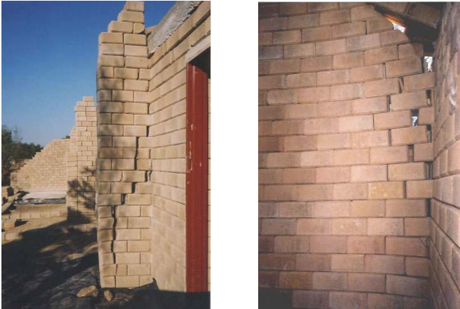
Fig 6-12: Buttress collapse, Hunts End
