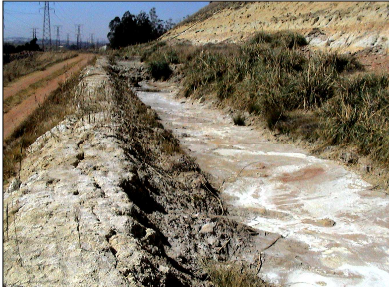
Figure 1.7b Efflorescence along a solution trench at Crown Mines (Nasrec dump) (Photograph by Tutu, 2005)
