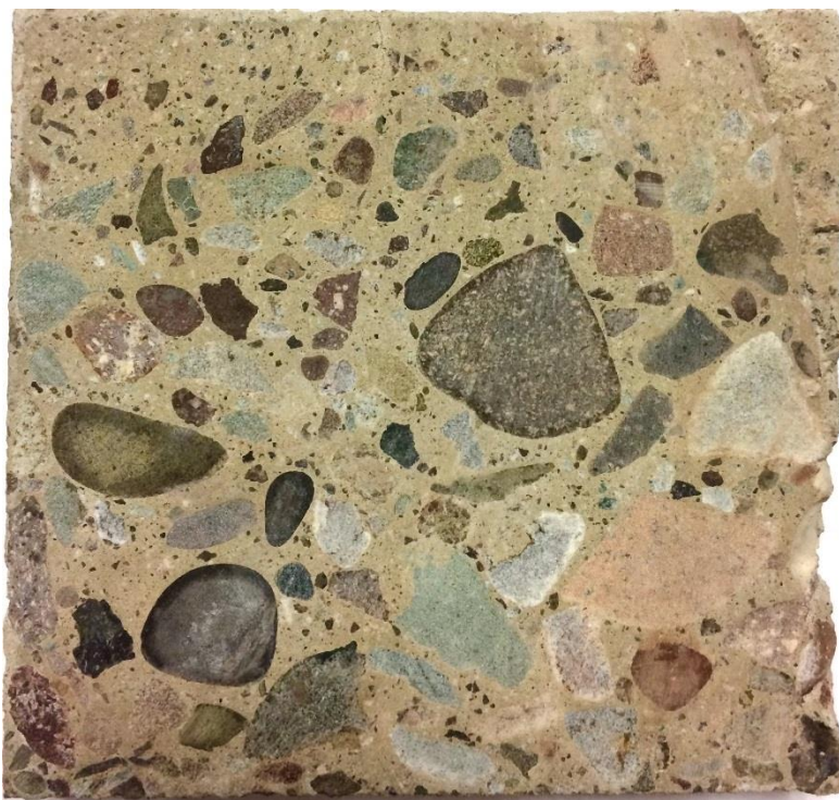
Figure 4-3 – T9 cross section showing aggregate segregation
