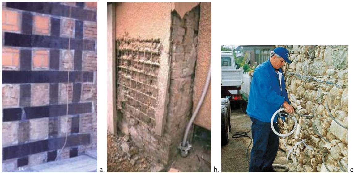
Figure 1: Examples of different methods to retrofit shear walls: a. Epoxy-bonded Carbon FRP, b. Steel mesh reinforced concrete jacketing, c. Grout Injection in the internal core of multi-leaf stone walls.
