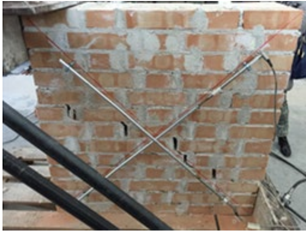
Figure 15: Typical diagonal cracking of control URM wall specimens.
