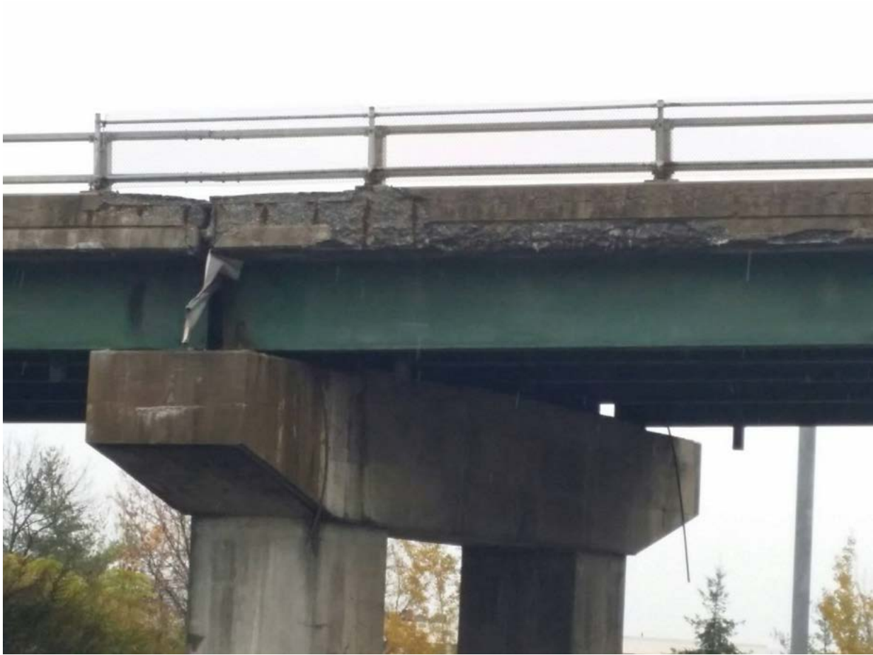
Figure 5.22 Closeup of Williston I-89 Overpass Tafts Corner with encasement repair of the pier, failed expansion joint gutter and distressed fascia
