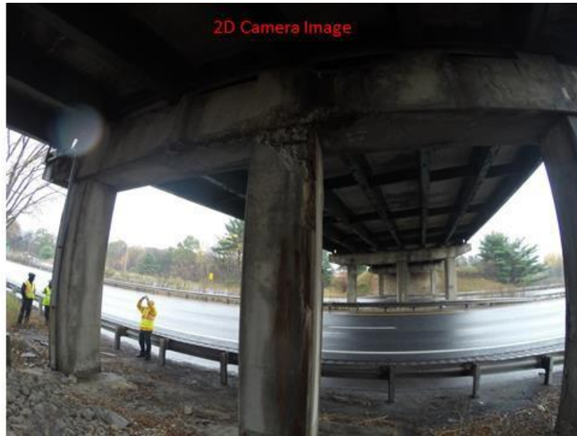
Figure 5.12 Spalling on column of Colchester/Milton I-89 Bridge
