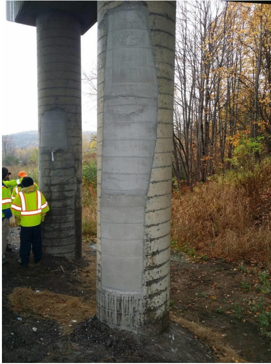
Figure 28: Patches on columns to fix spalling and cracking.
