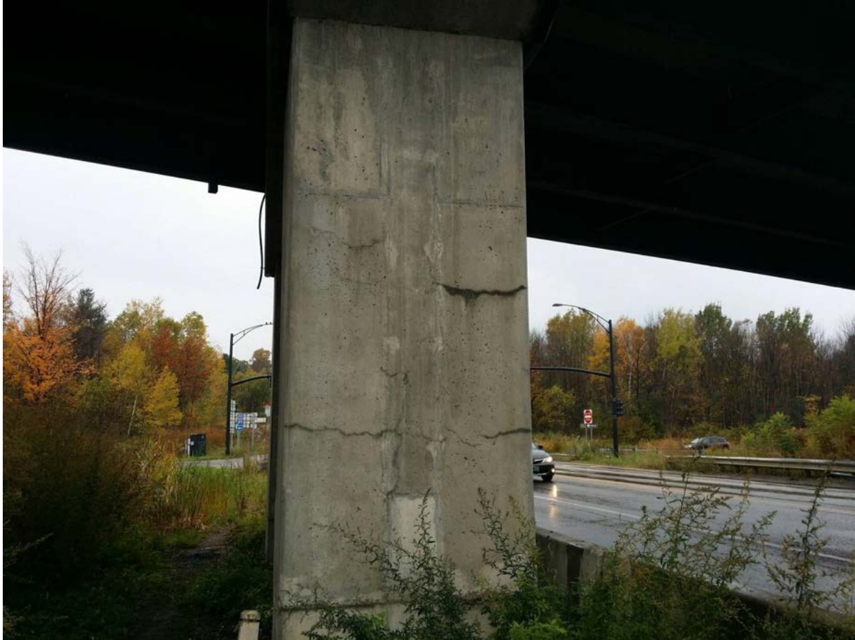
Figure 5.19 Encasement repaired column on Williston I-89 Overpass Tafts Corner, with visible cracking
