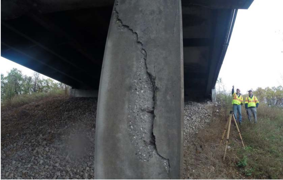
Figure 5.14 Column with distress on Colchester/Milton I-89 Bridge
