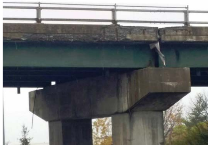
Figure 27: Spalling and steel corrosion on concrete fascia.
