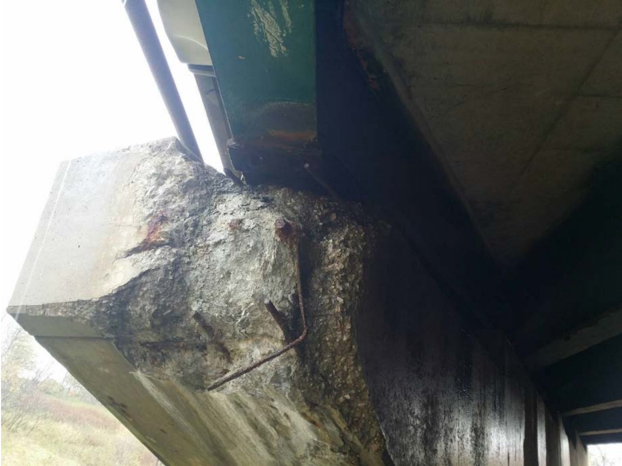
Figure 5.38 Close-up of pier cap with lost corner section leading to subsided bearing on Richmond I 89 US 2 Underpass Bridge
