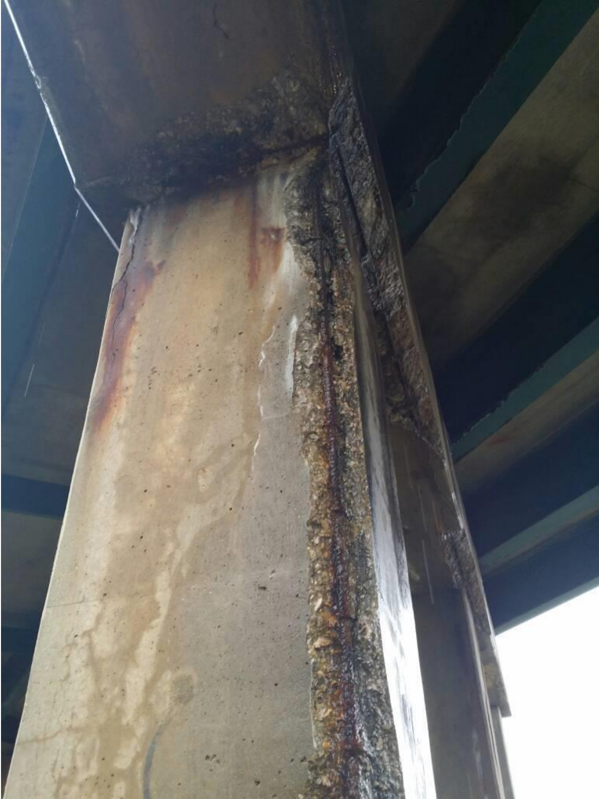
Figure 5.34 Square column with spalling at the corners and pier cap on Richmond I-89 US 2 Underpass Bridge
