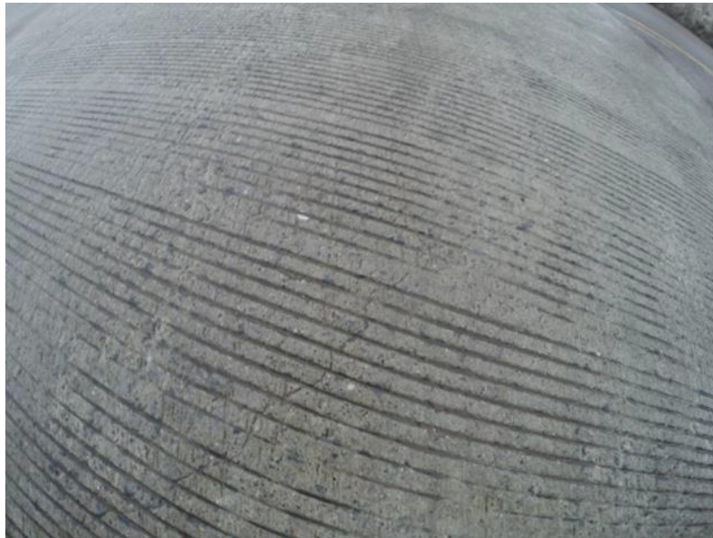
Figure 5.42 Deck patterned with cross-span cracks, approximately every 200 mm on Stowe Rte 100 Gold Brook Crossing Bridge
