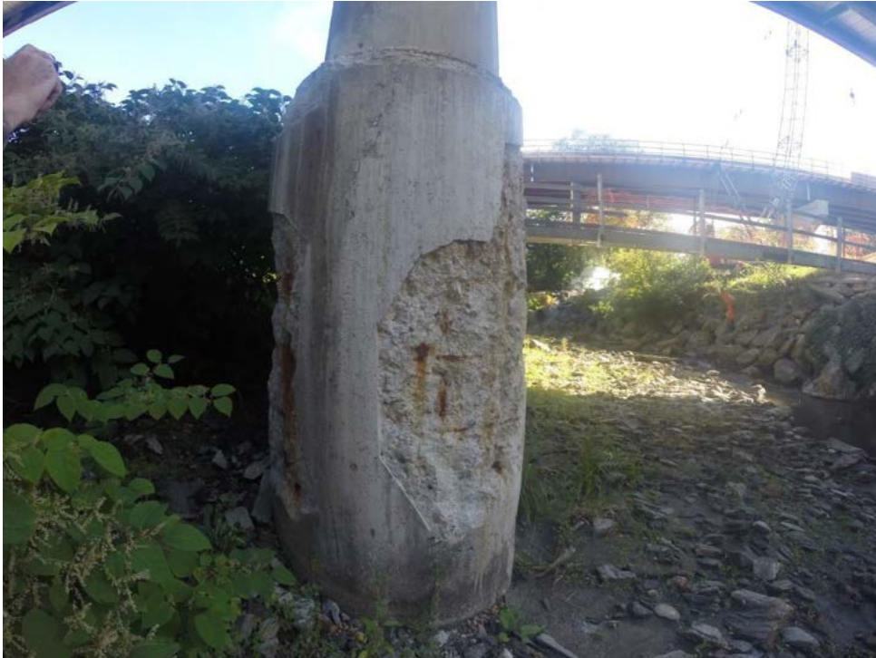
Figure 5.45 End view of pier base with damaged concrete removed on I-89 Waterbury Overpass Bridge
