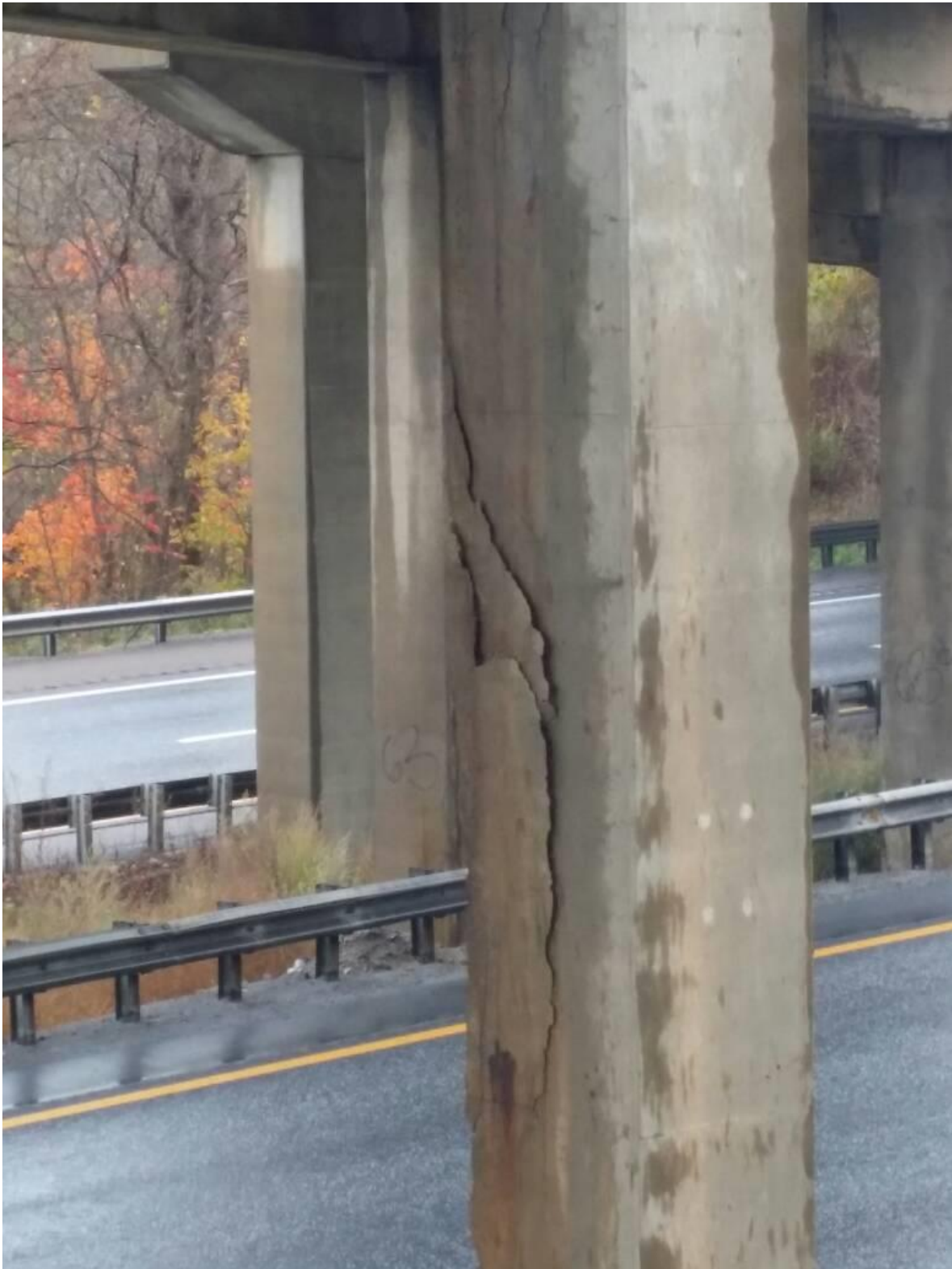
Figure 5.35 Column with spalling at the corners on Richmond I 89 US 2 Underpass Bridge
