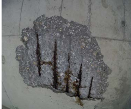
Figure 30: Spalling and slight steel reinforcement corrosion on underneath portion of concrete deck
