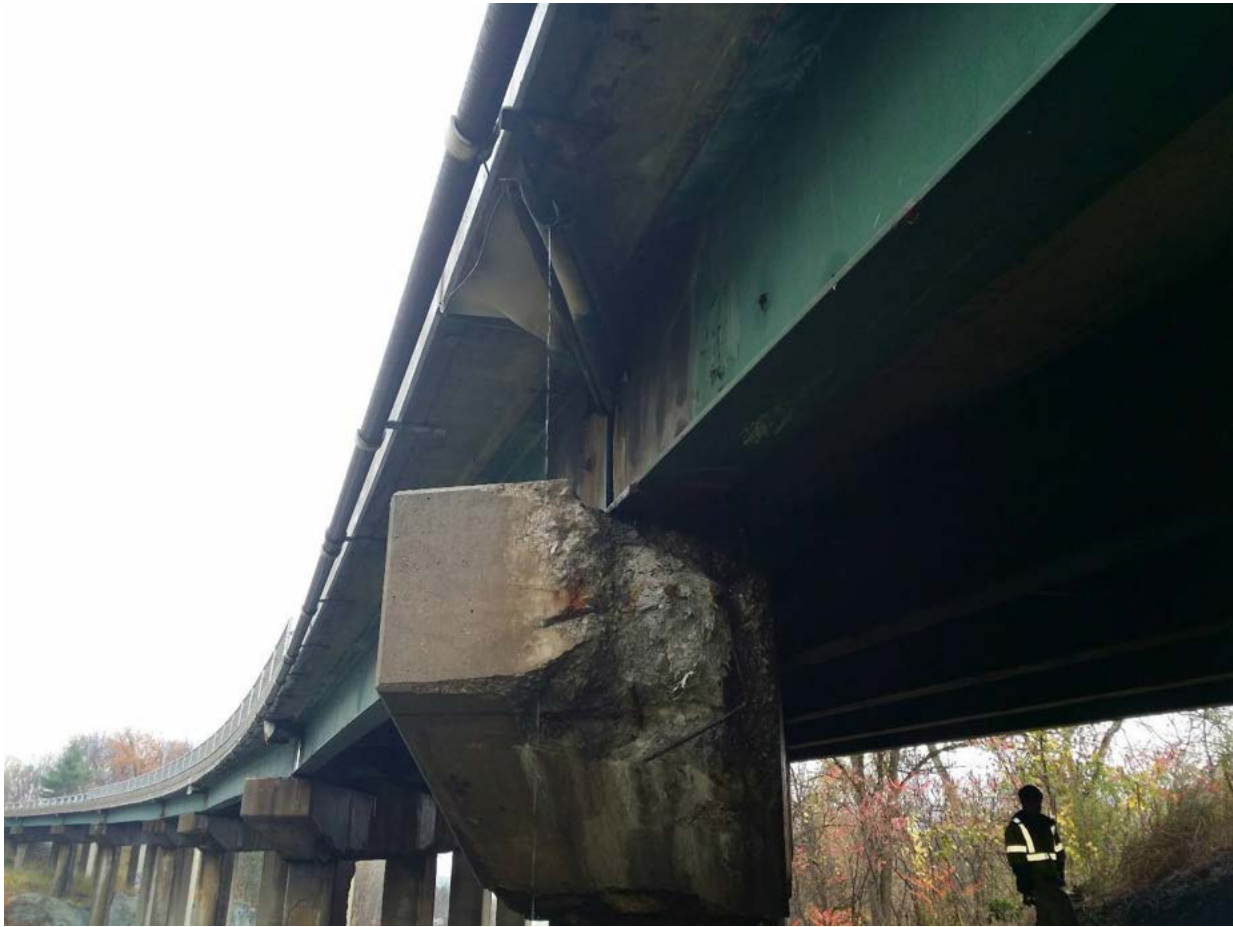
Figure 5.37 Pier cap with lost corner section leading to subsided bearing on Richmond I 89 US 2 Underpass Bridge
