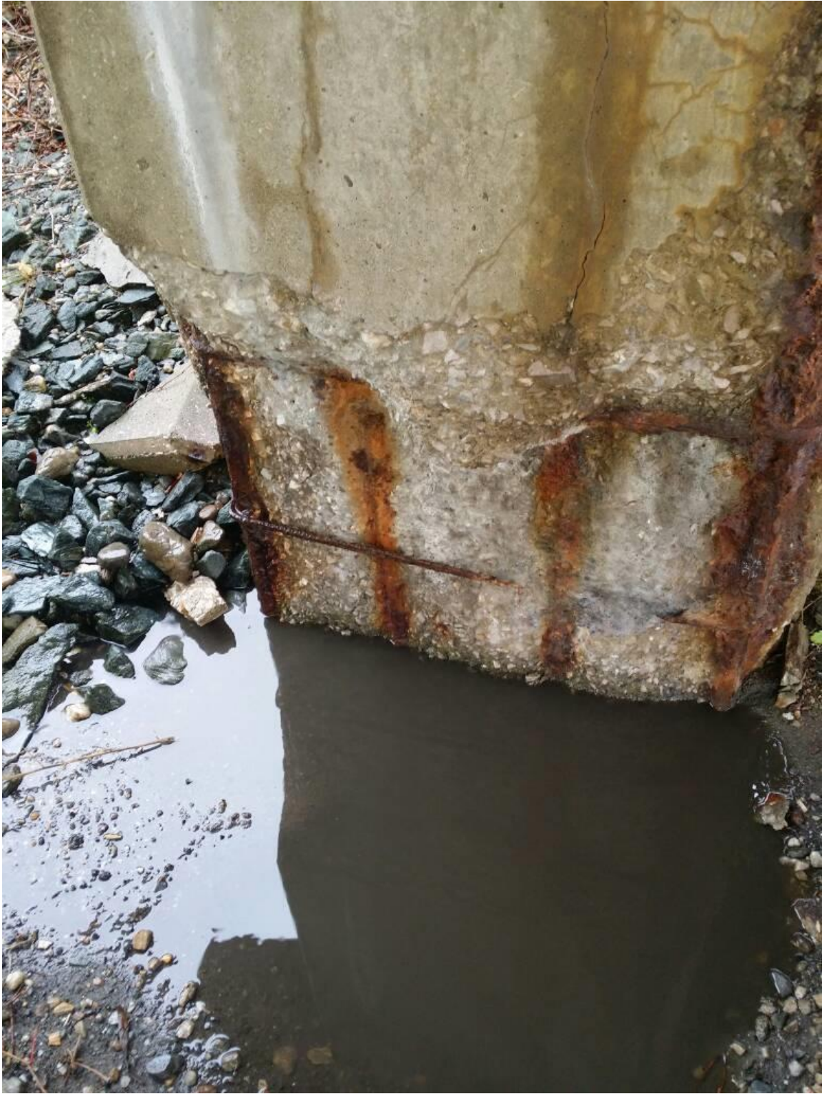
Figure 5.31 Distressed footing of a column on Richmond I-89 US 2 Underpass Bridge
