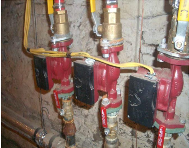
Grundfos multi-speed pumps. The switch on the center left of the black cover allows selection of one of three motor speeds resulting in variation of the flow.
