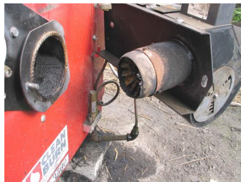
The nozzle and fan inside the burner tend to gunk up and must be cleaned regularly.
