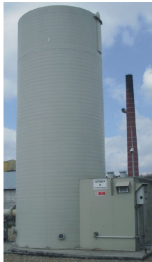
Figure 3. BG desulfurizer in the biogas plant in Liszkowo (photo B. Igliński).
