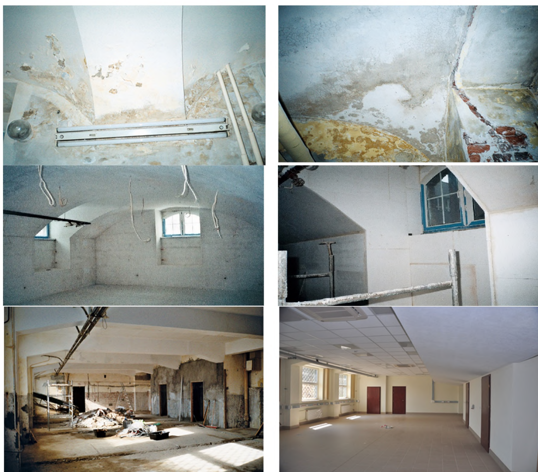
Figure 4. Photographs before, during and after the energy retrofitting process of selected cellar spaces.
