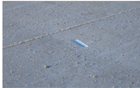
FIGURE 6: Popouts or mortar flaking [12].
