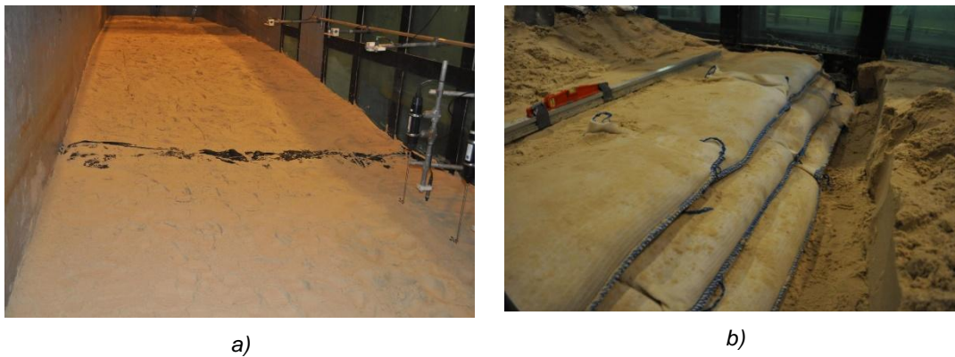
Figure 3. Images of the a) geotube installed in the beach and b) geobags during installation in the beach
