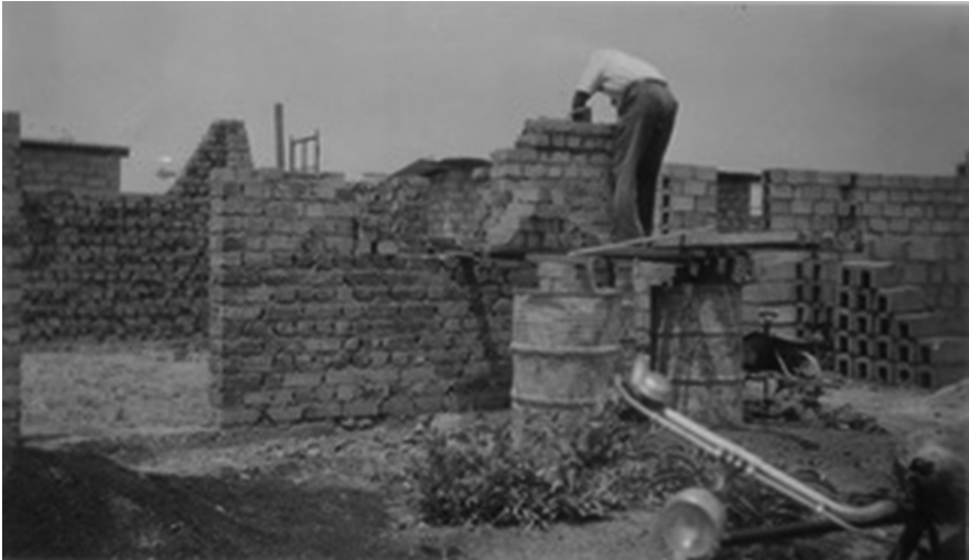
Figure 3.3: Building with the Système Grévisse in Lubumbashi. Source: Archives of the Soeurs de la Charité, Gent, file A 76-CON Lubumbashi.
