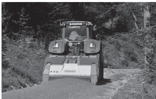
Fig. 1 »PTH Crusher 2500 HD« mounted on a Fendt 939 tractor crushing the windrowed ungraded material and leaving behind graded forest road surface layer material
