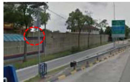
Figure 8. Holes present on wall barrier.
