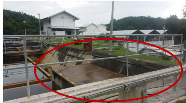
Figure 2. A structural crack was observed on the Water Sedimentation Plant storage tanks.
