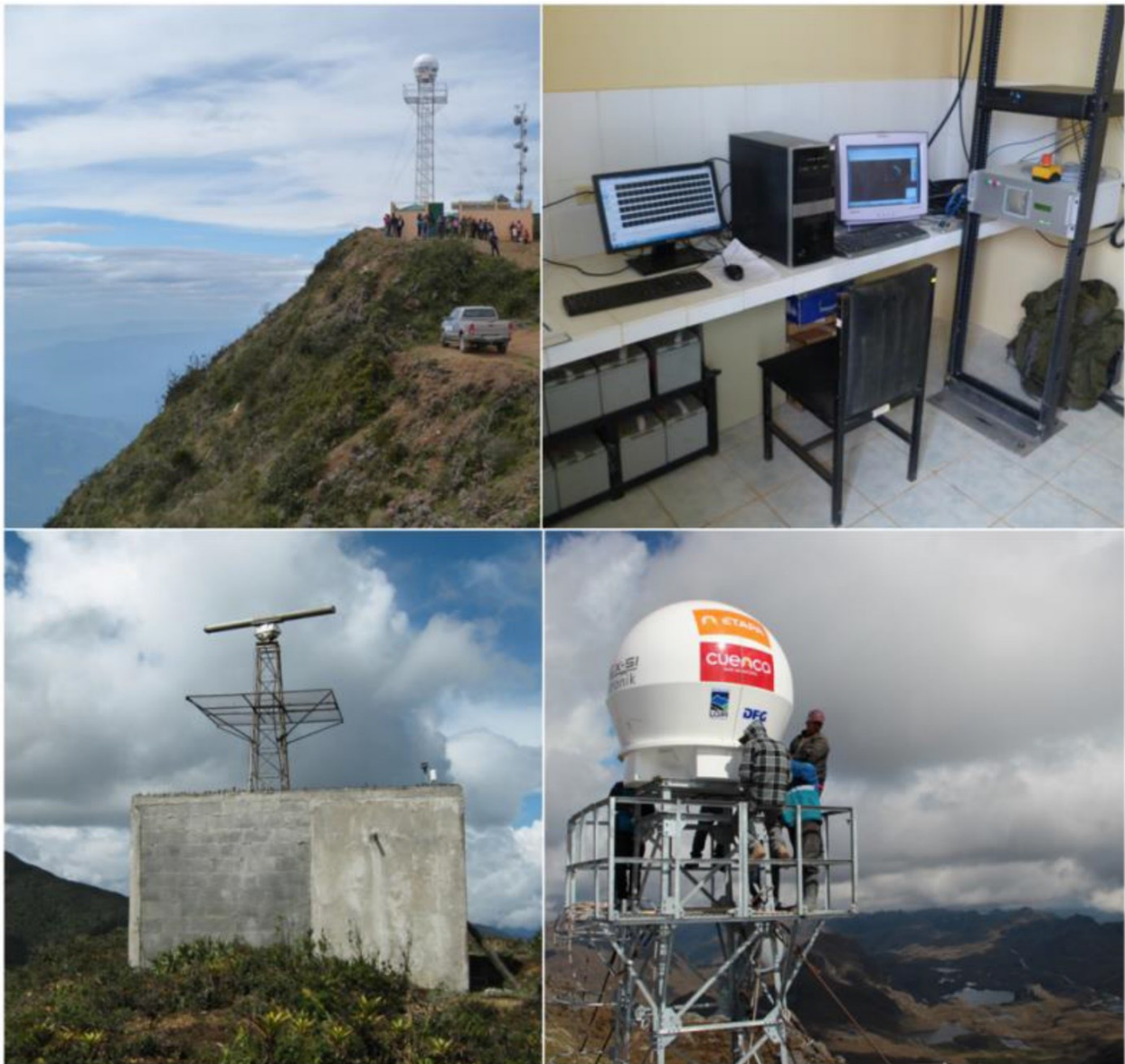
Figure 2.2: (top left) X-band scanning instruments of RadarNet-Sur: radar GUAXX RS120 RAINSCANNER on Cerro Guachaurco (3,100 m a.s.l.), (top right) GUAXX radar processing unit with backup power supply, (bottom left) radar LOXX LAWR at El Tiro (2850 m a.s.l.), and (bottom right) radar CAXX RS120 RAINSCANNER on Cerro Paragüillas (4450 m a.s.l.).
