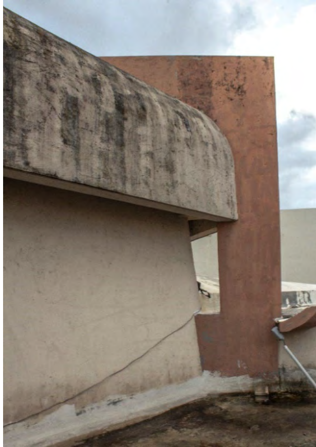
Fig. A2.73 – Discoloration, fouling and paint peeling conditions on Column A. Photo by Author, 2020.
