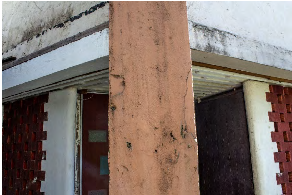
Fig. A2.80 – Scaling and fouling issues on Column C. Photo by Author, 2020.
