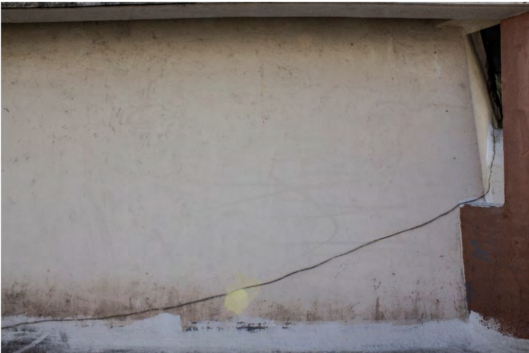
Figs. A2.54 & A2.55 – Horizontal and vertical highline cracks, minor detachment/debonding sections and scaling along the surfaces. Photos by Author, 2020
