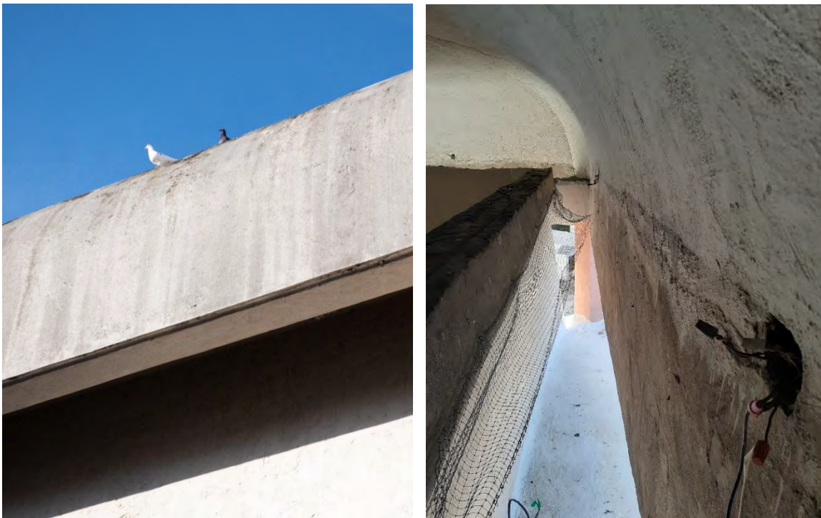
Figs. 4.26 & 4.27 – In the early 2010s the Church’s administration installed a pigeon netting along the dome. These nets are currently deteriorated. Photos by Javier Freytes, 2019 & Author, 2020.
