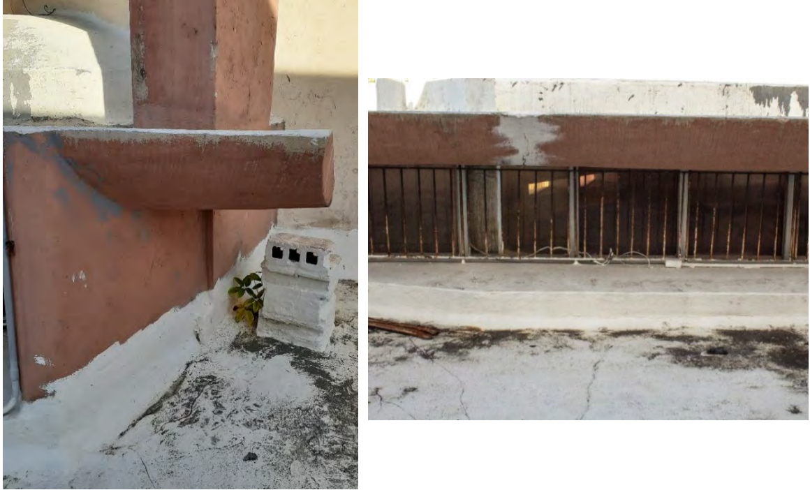
Figs. A2.44 & A2.45 – Major paint peeling, cracking and improper repairs in Elevation 10B. The sealing grey coating has also been applied to these concrete elements with a new paint coating of painting. Photos by Author, 2020.
