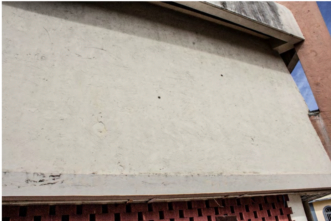
Fig. A2.63 & A2.64 – Large scaled stuccoed surfaces, fouling and guano issues on Elevation 15. Photos by Author, 2020
