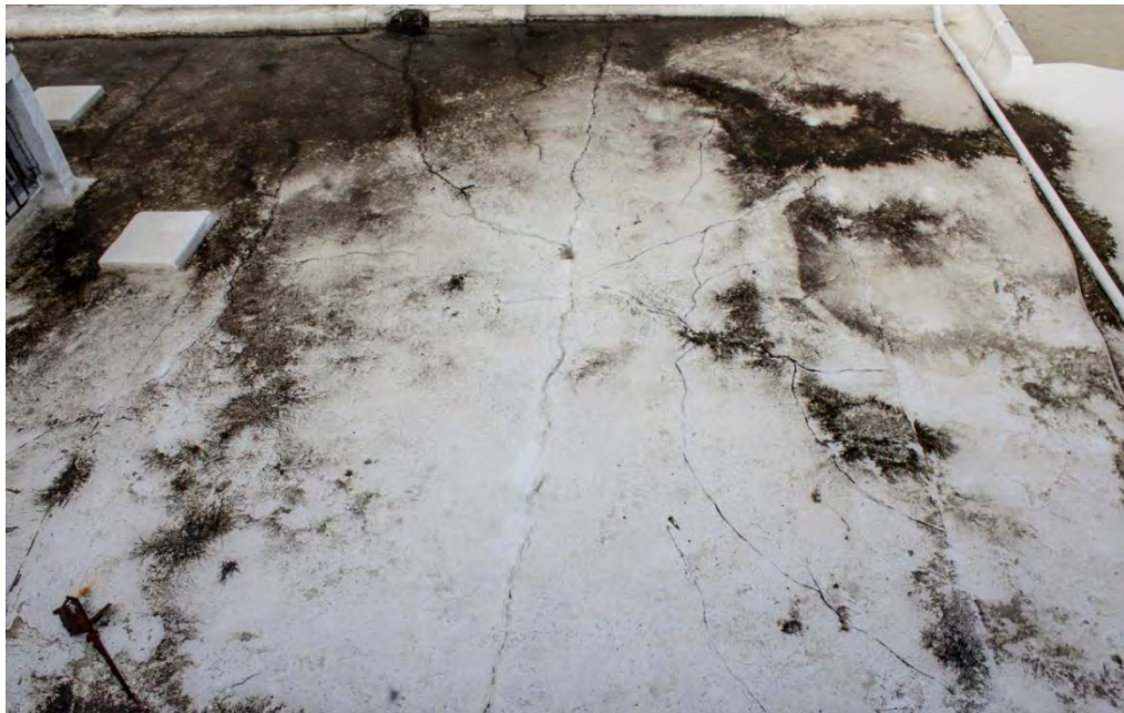
Fig. A2.37 – Current condition of the roof slabs on the west side of the church - Elevation 9. Photo by Author, 2020.
