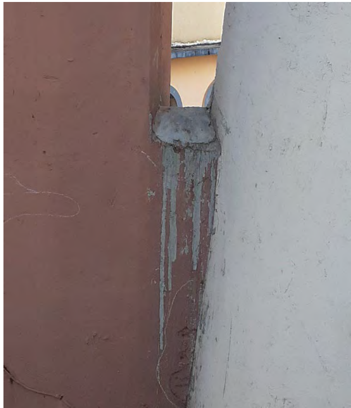
Fig. A2.94 – The installation of bird spikes with this silicone adhesive was used between the stuccoed surfaces of the tilted walls and columns C, D, E & F. Photo by Author, 2020.
