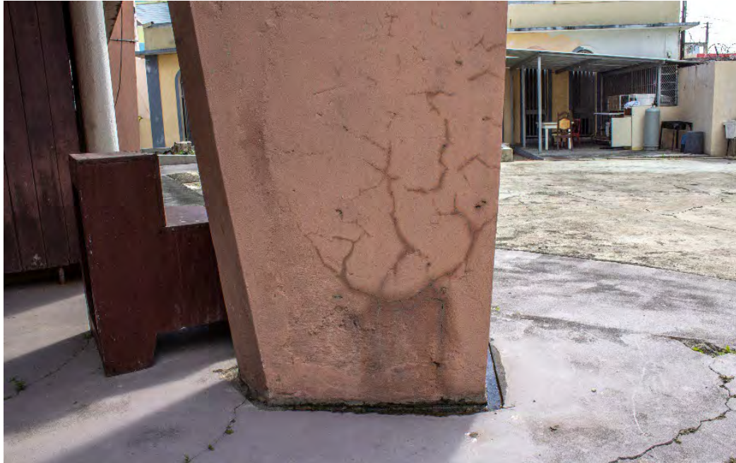
Fig. A2.84 – Possible alkali-aggregate reaction (AAR) on stucco (as defined by Poole & Sims, 2016) at the base of Column D. Common visual identification of this condition includes crazing surrounded by moisture and discoloration patterns, and efflorescence. Photo by Author, 2020.
