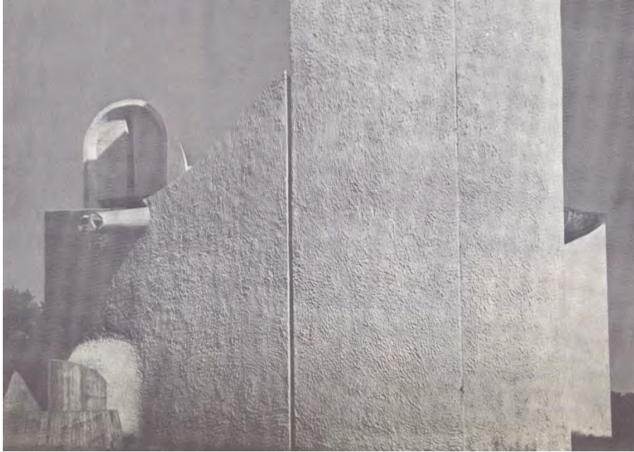
Fig. 2.43 – Photo of a Stuccoed Wall at the Notre Dame-du-haut Church at Ronchamp. Photo by Lucien Herve. Source: Manual of Lathering and Plastering by John R. Diehl, 1960.
