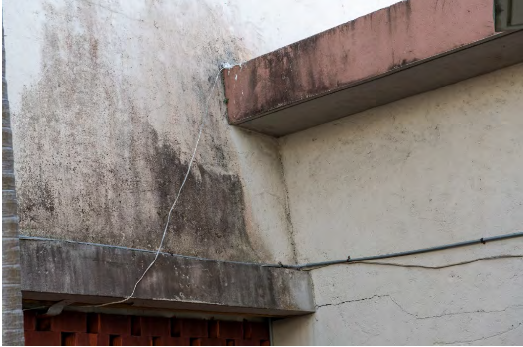
Fig. A2.53 – Bio-fouling growth and atmospheric soiling issues on the lower side of Elevation 12. Photos by Author, 2020.
