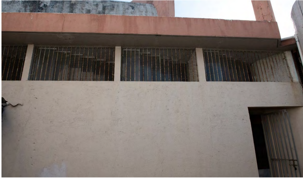
Fig. A2.29 – Slight vertical cracking, paint peeling and soiling issues on the eaves of Elevation 7. Photos by Author, 2020.
