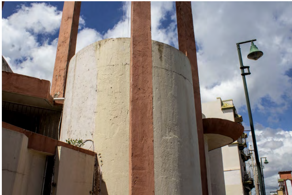
Fig. A2.9 – In elevation 3 two different paint coating applications can be found. A horizontal continuous slight crack along the concrete masonry wall show signs of steel reinforced corrosion. A vertical crack stained by mold is also seen on the top part of Side A. Photos by Author, 2020.
