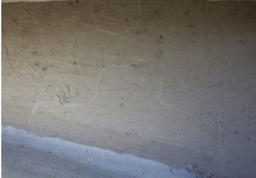
Fig. A2.34 –Detaching/debonding areas with small hairline diagonal cracks on the stuccoed tilted wall on Elevation 8. Photos by Author, 2020.
