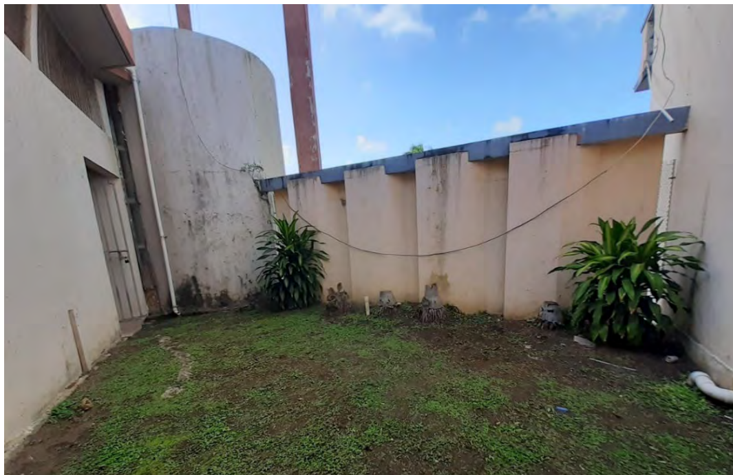
Fig. A2.22 – Remaining palm trees and other large leafy plants close contact with the precast panels. The original paint from the church's exterior surfaces is also visible from this side. Photo by Javier Freytes, 2019.
