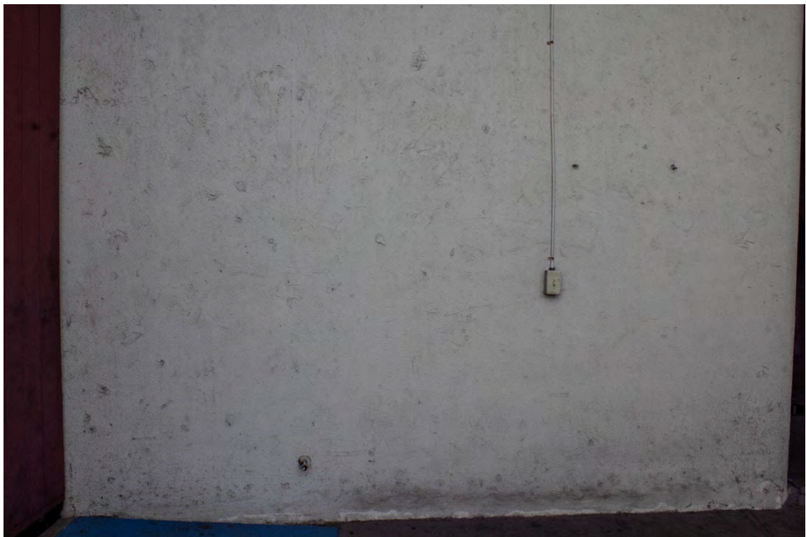
Fig. A2.14 – Major scaling, rinsing damp and paint peeling issues can be seen in Elevation 4. Photo by Author, 2020.
