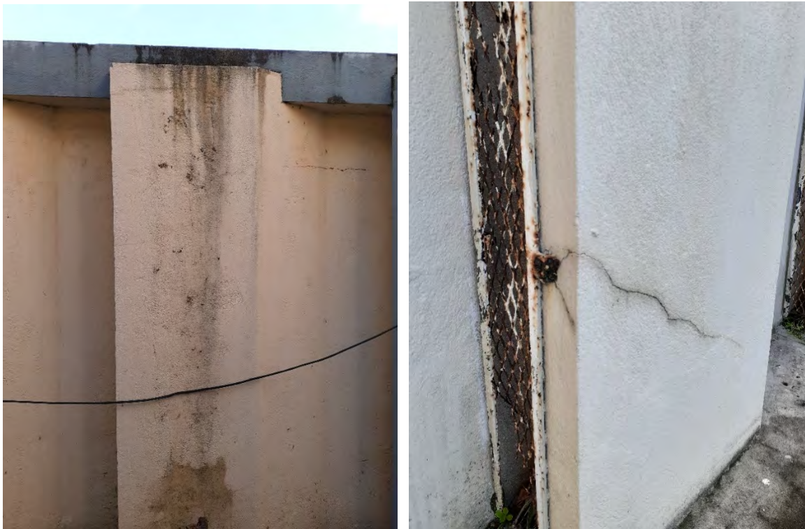
Fig. A2.24 & A2.25 –Soiling and mold issues on the surfaces of the precast panels on Side B (left photo). Diagonal slight cracking due to steel corrosion on Side A of the precast panels (right photo). Photos by Author, 2020.
