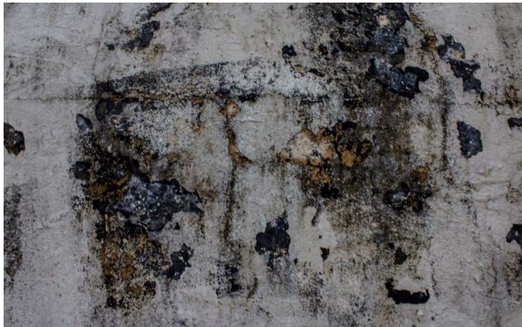
Fig. A2.35 – Vertical and horizontal microcracking, paint peeling and moisture issues on the surfaces of the dome on Elevation 8. Photo by Author, 2020.
