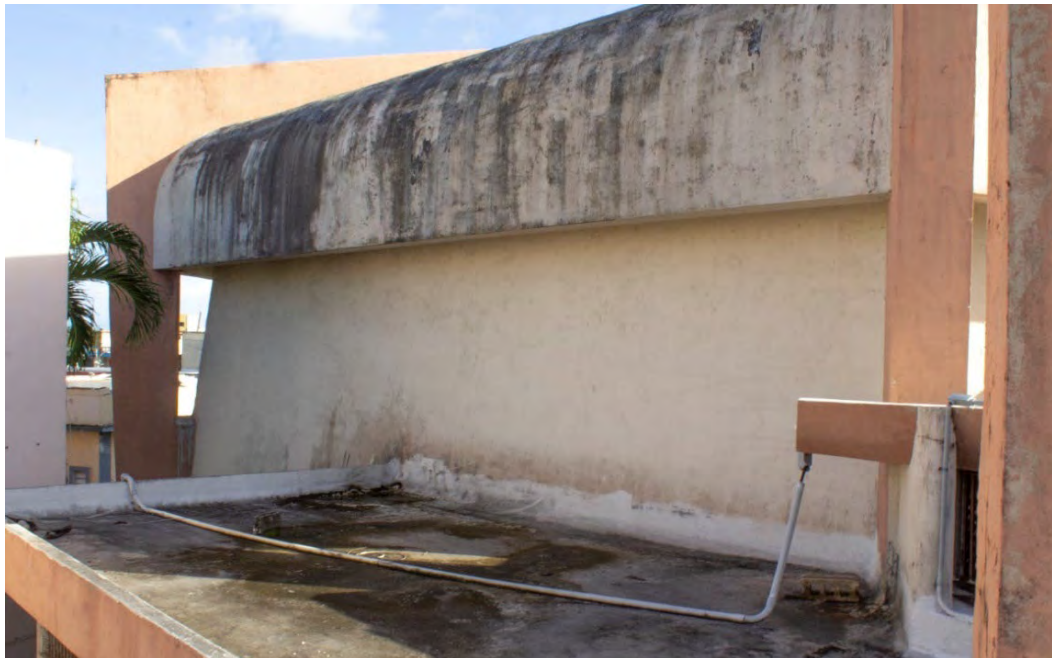
Fig. A2.52 – The application of a sealing coating to the stuccoed wall is causing moisture, bio-fouling and discoloration issues. Photos by Author, 2020.
