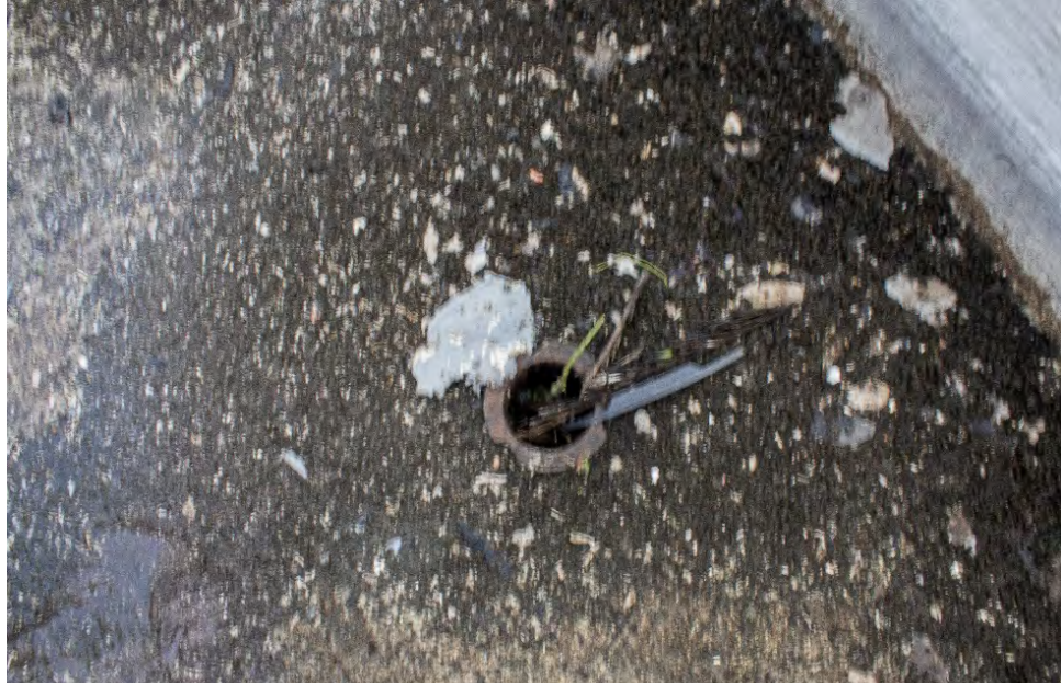
Fig. A2.38 – Broken 'Type A' original roof drainage on roof slab near baptistry and confessionary – East side (bottom photo). Photo by Author, 2020
