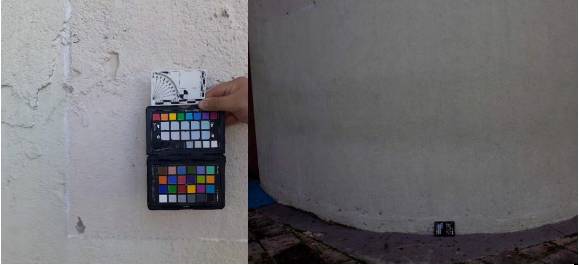
Figs. A2.2 & A2.3 – Scaling and rising damp issues on Elevation 1. As the main entrance to the church, a big sign was originally installed using screws and eventually removed. At least two paint coatings could be identified in the wall. Photos by Author, 2020.
