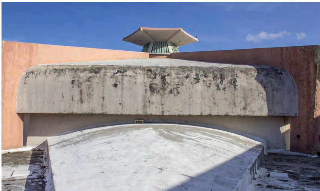
Fig. A2.33 – Surface fouling and paint peeling/deterioration on Elevation 8 (top photo). Photo by Author, 2020.
