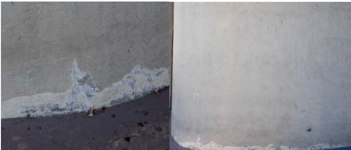
Figs. A2.4 & A2.5 – Rising damp, discoloration and paint peeling issues on Elevation 2. Photos by Author, 2020.
