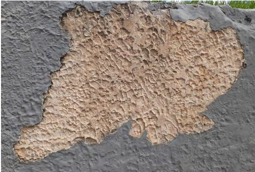
Fig. 3.6 – Photo of the original "Stippled Cement Plaster Finish" at the entrance of the UPR Museum of History, Anthropology and Art designed by Klumb in 1948. Photo by Author, 2018.
