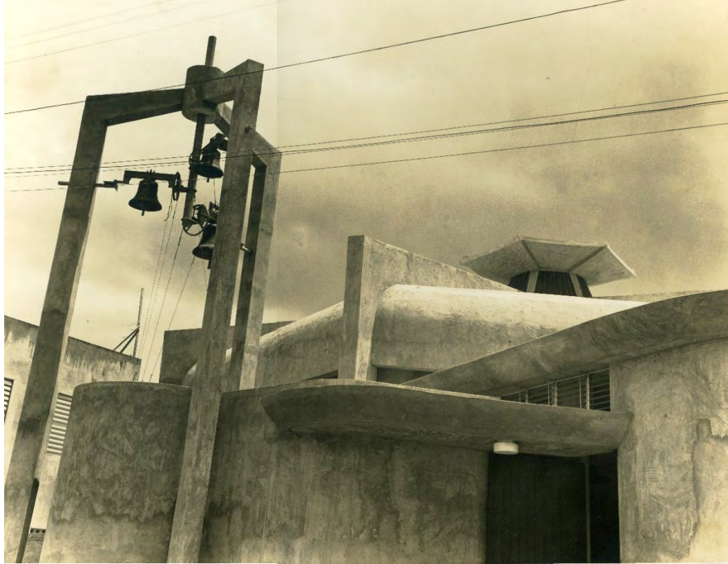
Fig. 2.36 – Details of the original exterior stuccoed surfaces on the northeast side of the church, c.1963. Source: AACUPR – Henry Klumb Collection.
