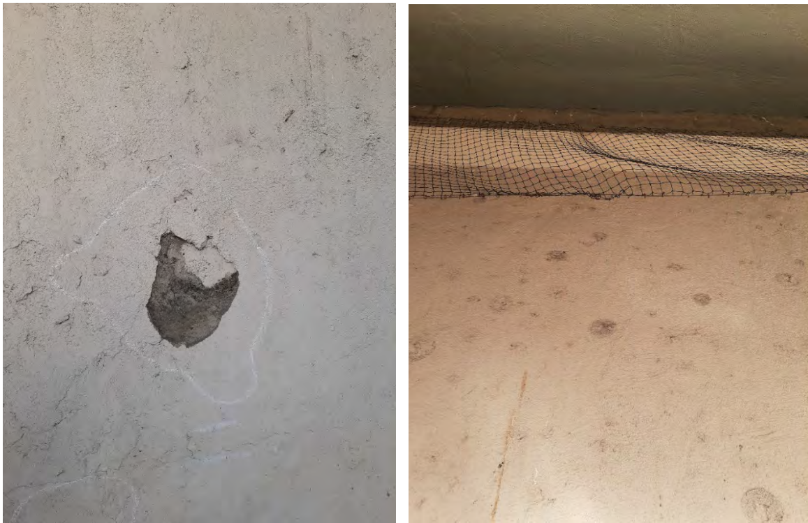
Fig. A2.66 & A2.67 – Elevation 16 showed some scaling and detachment/debonding conditions. Fouling and deterioration under the stucco layer is particularly visible in this section of the Elevation (left photo). Guano and soiling issues on the wall and a broken pigeon netting (right photo). Photo by Author, 2020.
