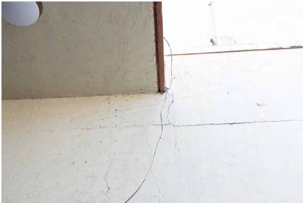
Figs. A2.15, A2.16 & A2.17- Scaling along detachment/debonding and discoloration of stucco near the entrance in Elevation 4 (top left photo). Macro biogrowth and development of vertical and horizontal slight/hairline as sign of reinforced corrosion on Elevation 5 (top right and bottom photos). Photos by Author, 2020.
