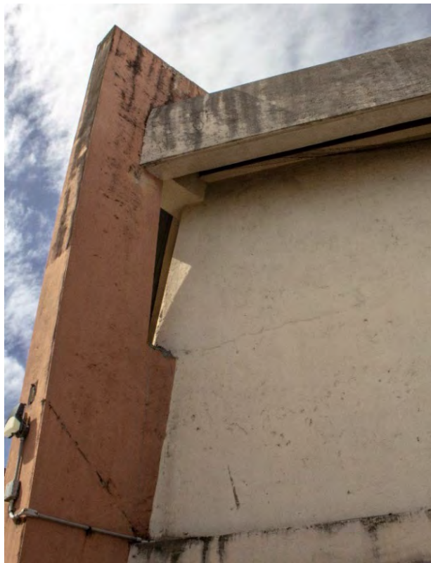
Fig. A2.61 – A diagonal slight crack and soiling are among the conditions in Elevation 14. Photos by Author, 2020.
