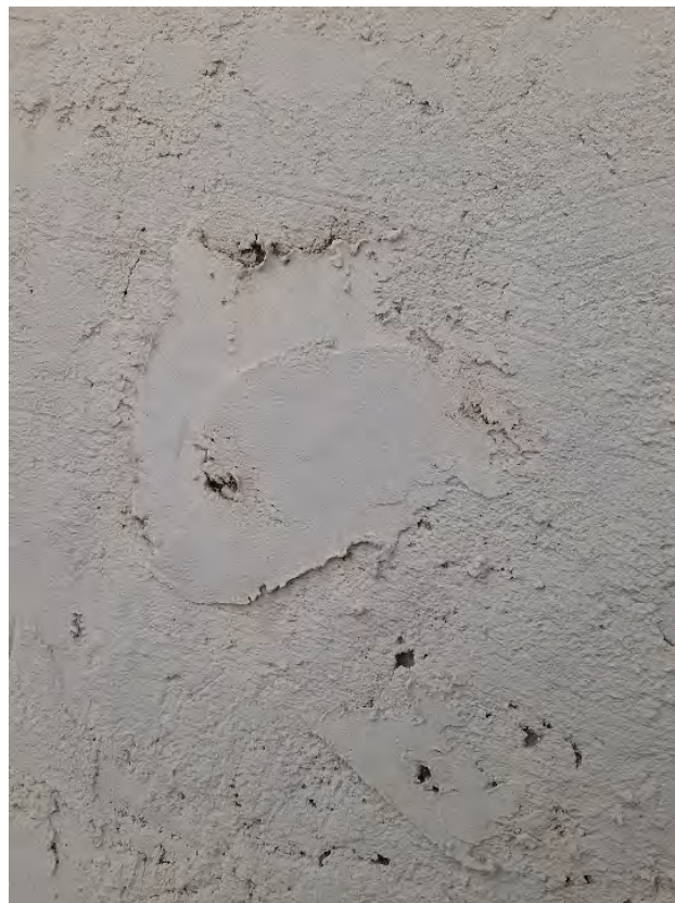
Figs. A2.57, A2.58 & A2.59 – Highline cracks along discoloration sections and scaled portions of the stucco in Elevation 13 (top photos). Original stucco patches -now covered- show the uneven workmanship over the exposed surfaces. Photos by Author, 2020.
