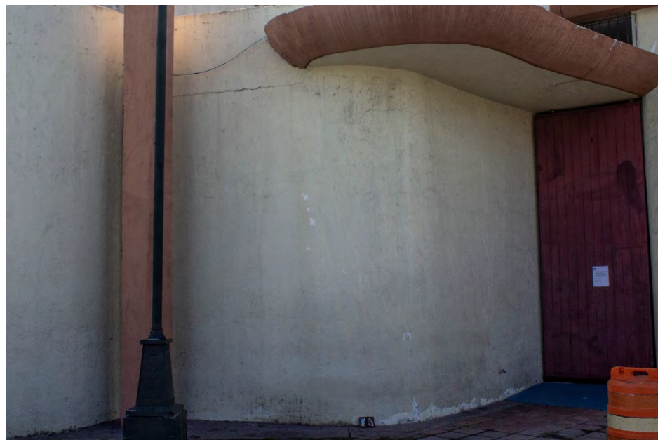
Figs. A2.6 & A2.7 – The wall is also affected by a small drainage in the curved eave which manage rainwater directly to the wall and concrete floor. A continuous horizontal crack in the wall surface is a sign of steel reinforce corrosion on the concrete masonry. Photos by Author, 2020.
