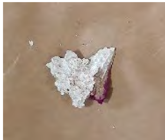
After the application of Phenolphthalein ( C_{20}H_{14}O_4 ) indicator – Results: No Carbonation
