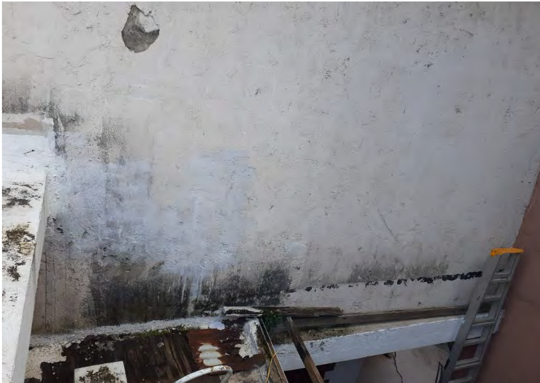
Figs. A2.68 & A2.69 – Cracking, scaling, guano, mold growth, fouling and moisture issues on Elevation 16. The roof sealing and waterproof coating was also applied to the base of the wall. Photo by Author, 2020.
