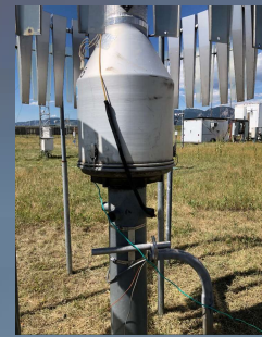
Figure 8. Photograph of The outdoor control with the grounding wire
