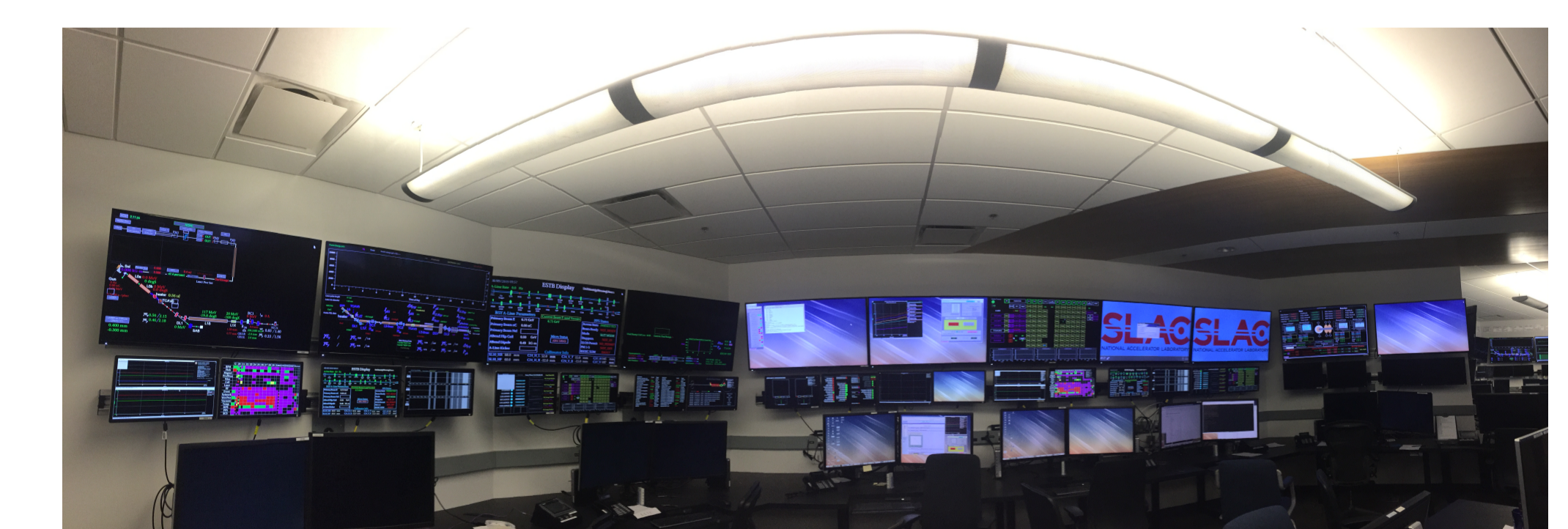
Figure 7: Accelerator Control Room, Building 52.
