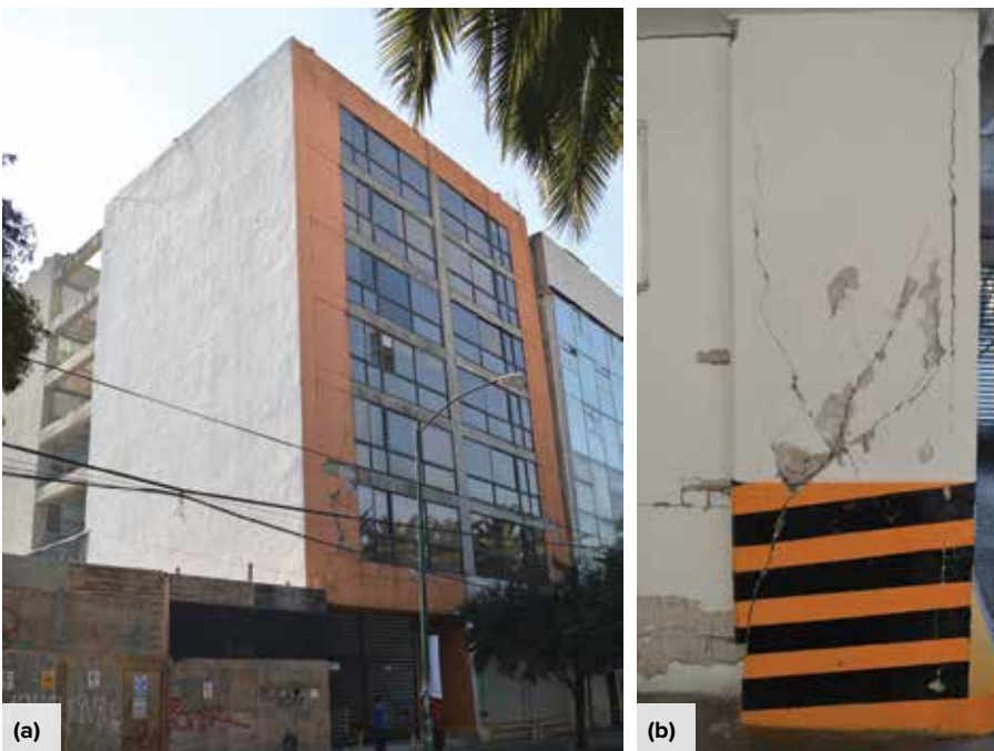
Fig. 6: A typical residential building affected by the 2017 Puebla Earthquake: (a) edge frames oriented perpendicular to the street had continuous infill walls and exhibited no significant damage; and (b) edge frames oriented parallel to the street had infill walls and fenestration and exhibited shear failure in first-story columns (after Reference 26, licensed under CC BY-NC-SA 4.0)
