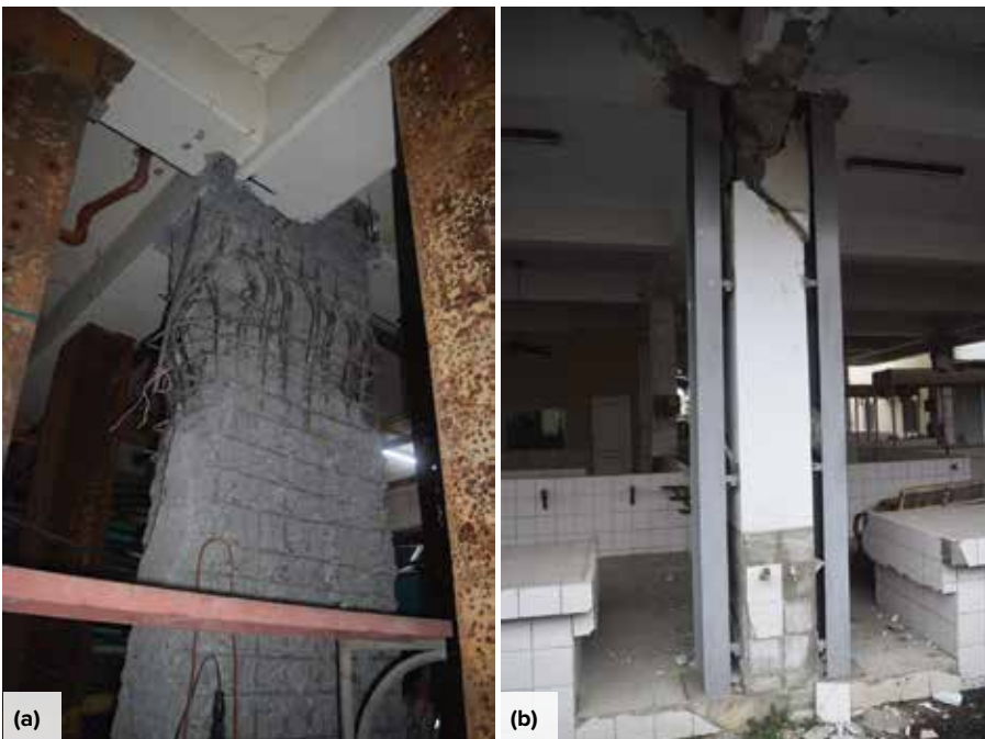
Fig. 4: Damage to columns in the 2016 Taiwan Earthquake: (a) axial compression failure; and (b) shear failure (after Reference 22, licensed under CC BY-NC-SA 4.0)
