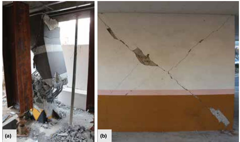
Fig. 7: Observed damage to RC structures in the 2017 Pohang Earthquake: (a) a first-story column; and (b) a structural wall in another building (after Reference 28, licensed under CC BY 3.0)
