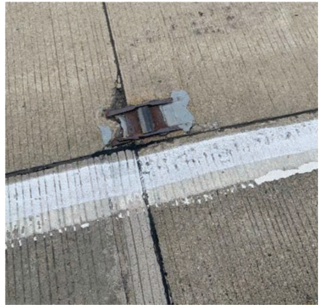
Figure 3.6 Damage to the longitudinal joints caused by RPMs (West Lafayette, IN-US 52).
