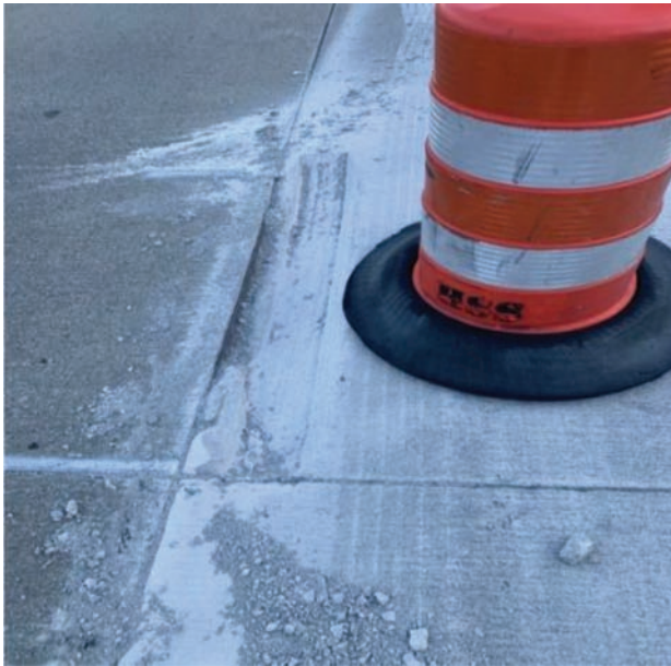
Figure 3.5 Damage to the longitudinal joints caused by removal of RPMs (Lafayette, IN-US 231).
