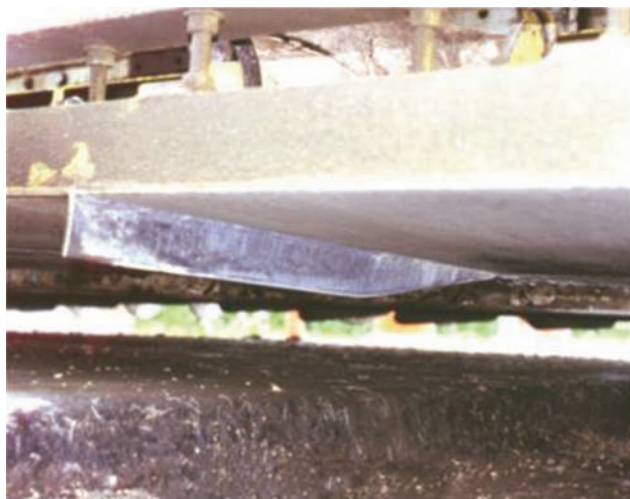
Figure 5.1 An early prototype of the joint-forming knife mounted to the bottom of the paver pan (Bergeron, 2004a).
