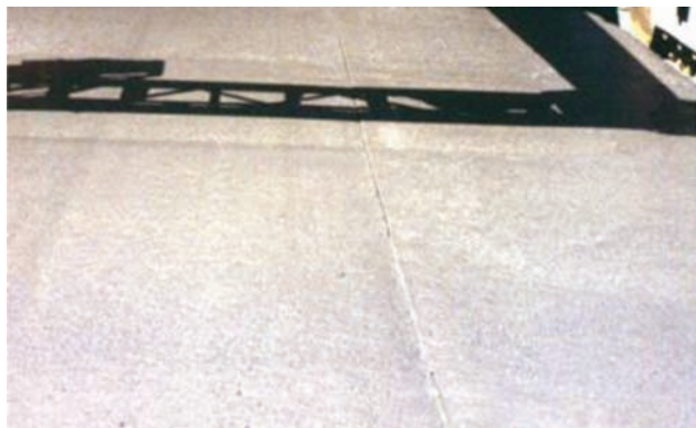
Figure 5.2 View of the formed joint behind the paver. After hand finishing, the joint becomes much less visible (Bergeron, 2004b).
