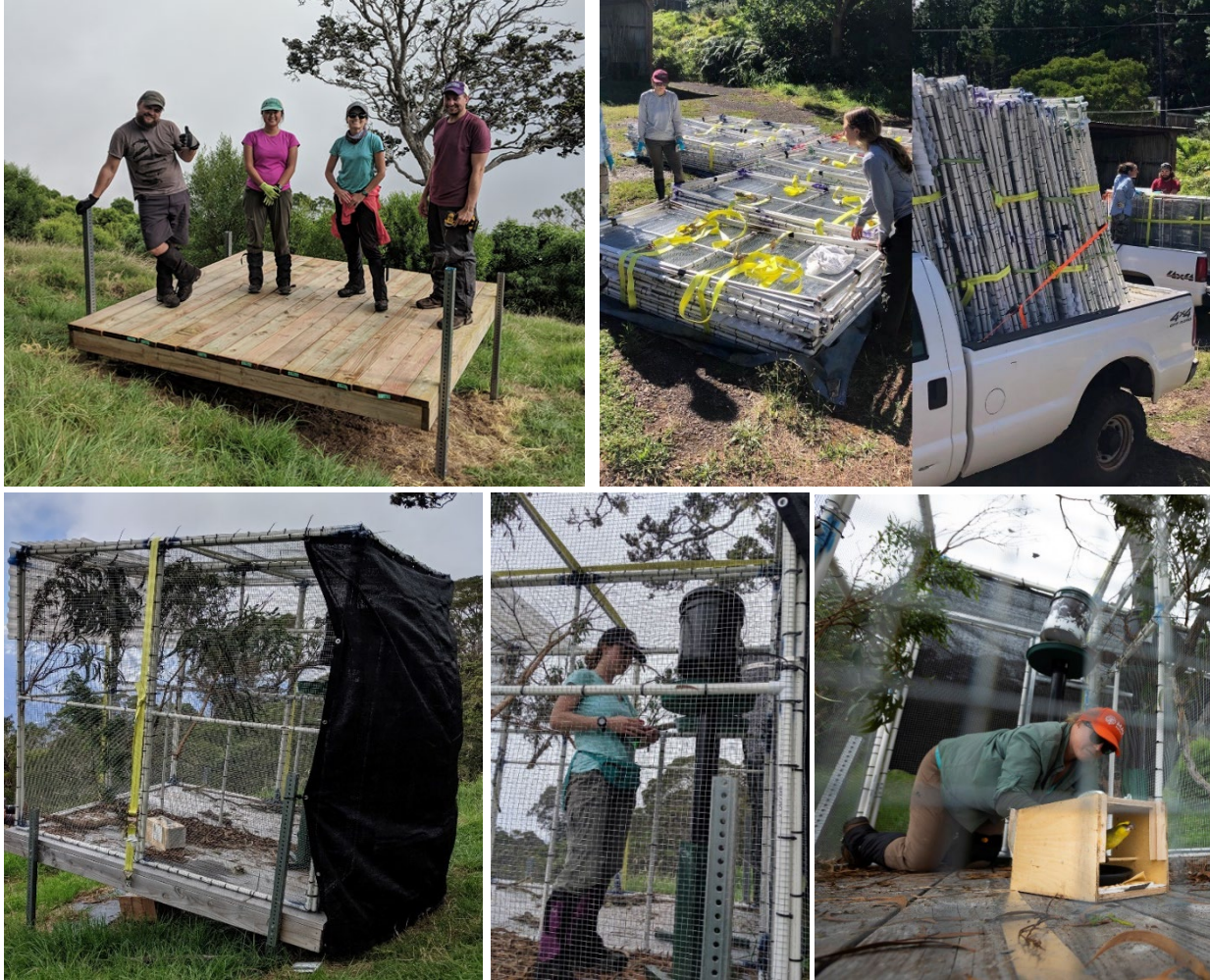
Figure 6. Photos (from left to right, top to bottom): Wooden platform, transport of aviaries in bundles to helicopter pick up site, completed aviaries in Nakula Natural Area Reserve, installing a supplemental feeder, and release of a kiwikiu to an aviary from transfer box.
