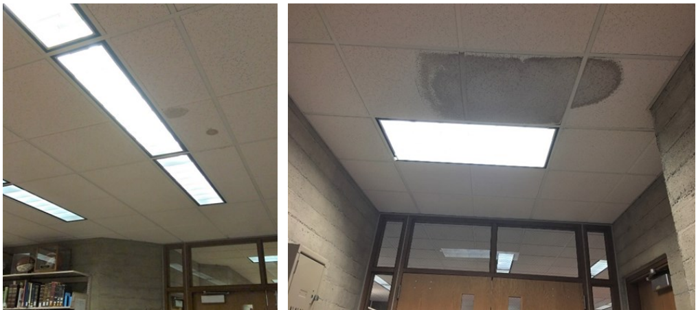
Figures 2 and 3. Ceiling leak in CWU Archives, October 2017 (left). Ceiling leak in CWU Archives, December 2017 (right).
