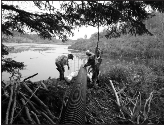
Figure 3. Installation of a pond-leveling device used to maintain water in beaver ( Castor canadensis ) ponds at constant levels. The pipe is placed in the beaver dam at the same level as the desired level of the pond, while the cage protects the end of the pipe from beavers. When water levels rise, water automatically draws through the pipe until reaching the level of the pipe through the beaver dam (photo courtesy of G. Hood).
