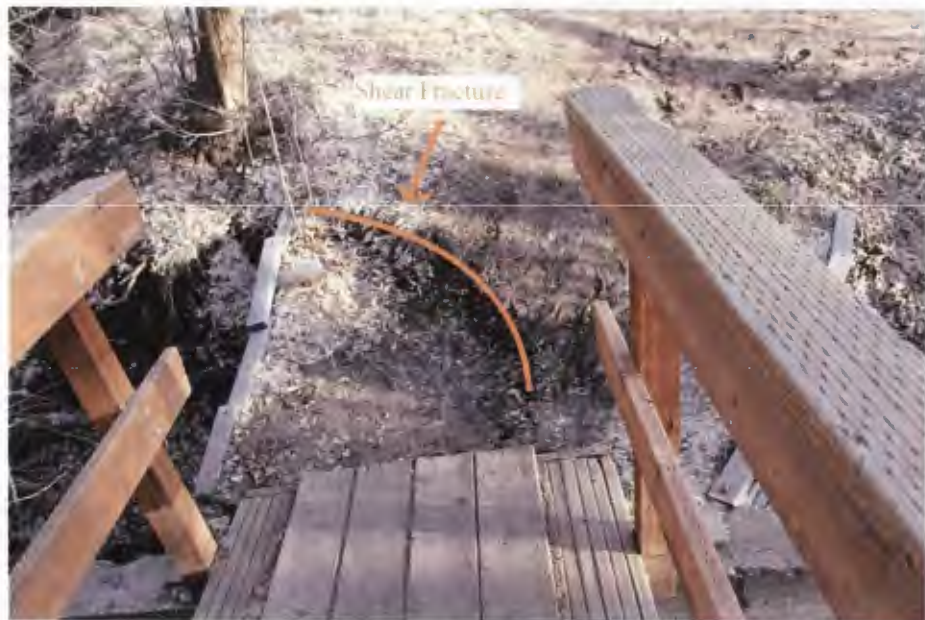
Figure 26. Footing shear failure.
