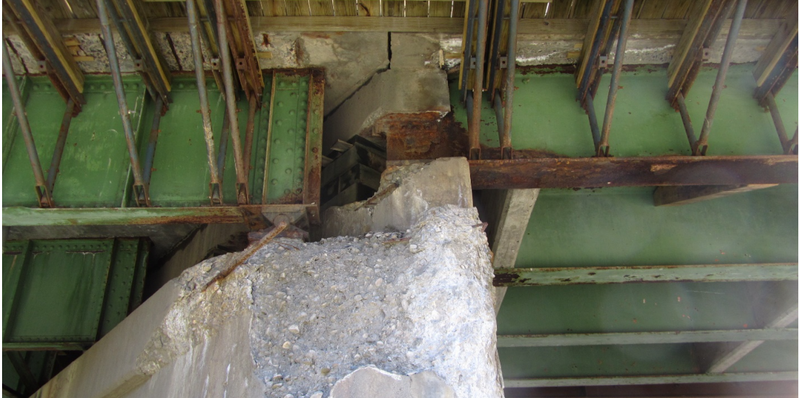
Figure 5.2: Example of an Aging Bridges in a Deteriorated Condition with More Corrosion
