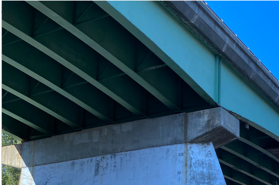
Figure 5.1: Example of an Aging Bridges in Good Condition with Slight Corrosion
