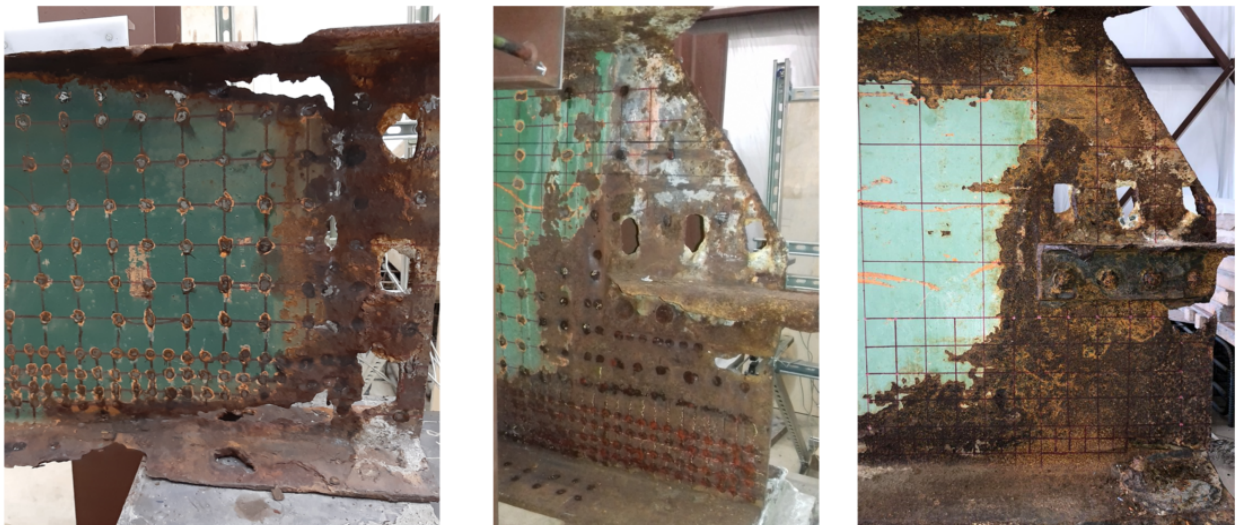
Figure 5.4: Corroded Girder Ends Extracted from Decommissioned Bridges. Points Along the Grids Indicate Locations where Paint has been Removed in Order to Obtain Thickness Measurements [52].
