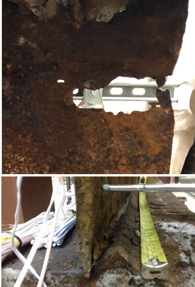
Figure 3.9: (Top) 4"x2" hole under end diaphragm; (Bottom) Initial Out-of-Alignment and Web-Flange Discontinuity.
