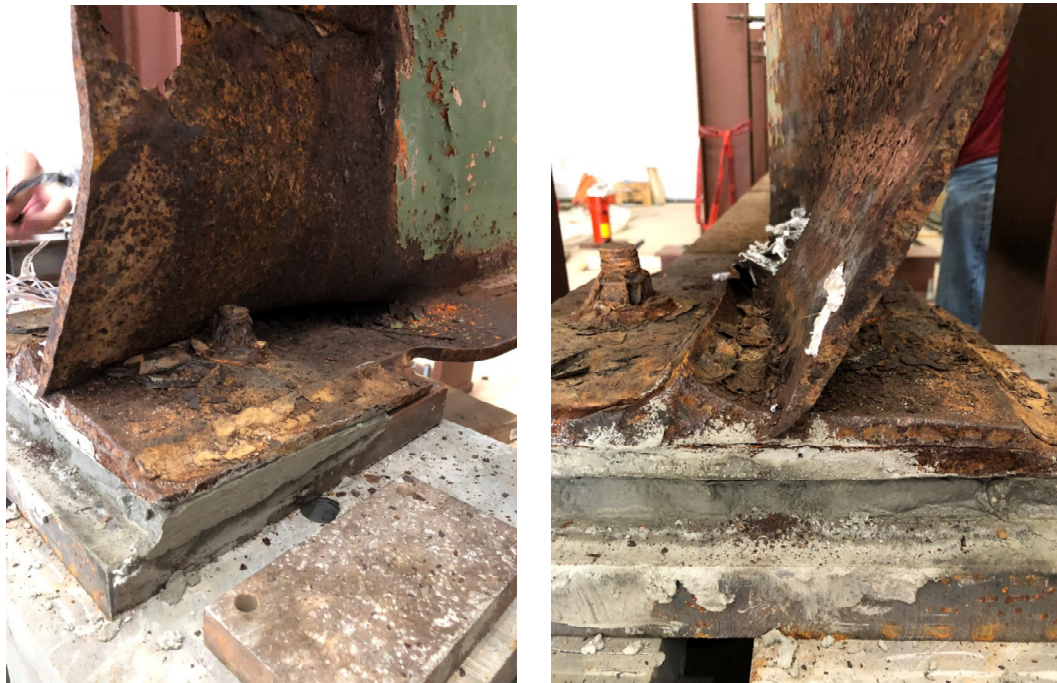
Figure 4.9: Residual Deformation of Corroded Web End
