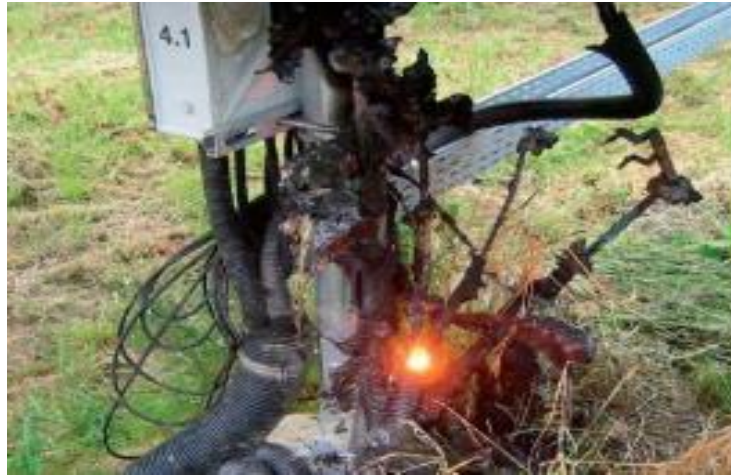
Figure 4: Arcing persists in the DC wiring even after a fire consumes a portion of the combiner box [4].
