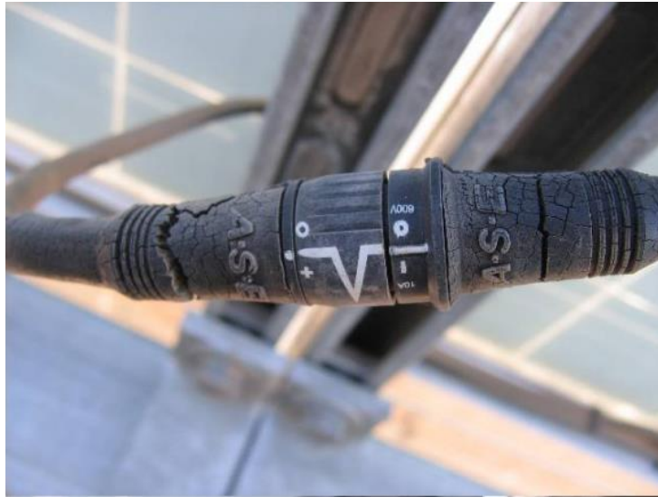
Figure 3: An example of aging cable connectors which are very likely to cause loose connection [3].
