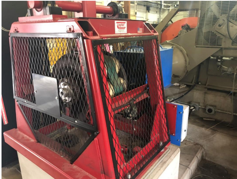
Figure 10: Taylor DAE150 connected to Ajax E-565
