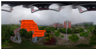
FIGURE 16 An image not separated into subimages is evaluated by PADENet. The majority of defects are correctly detected, leaving only some small-scale damage unclassified.
