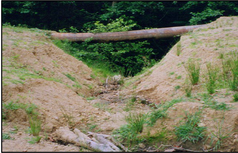
Figure 1.4 – Free Spanning Pipe Due to Soil Erosion (Georgia)
